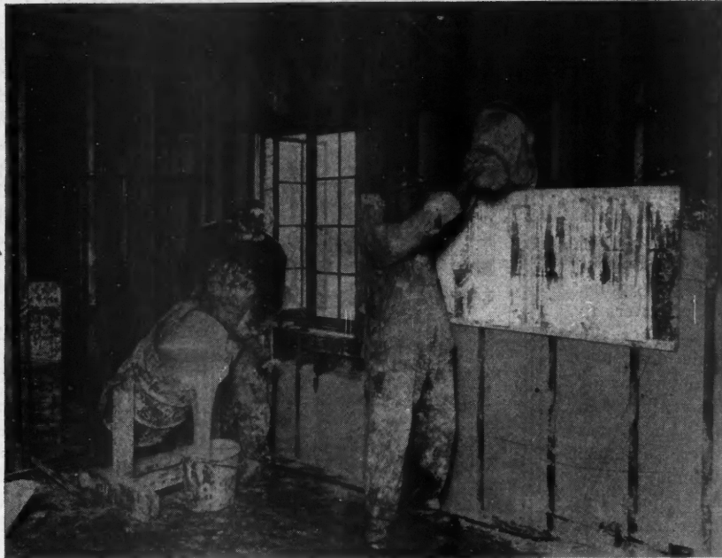
Bulk Insulation Is Poured Between the Studs and Held in Place by Means of Light Forms Until It Has Set, Which Requires about 30 Minutes.
