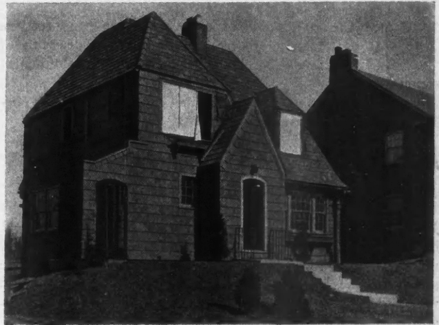
After the Fire—Note that the Exterior Is Undamaged Although the Inside Was Burned Out Clean. Gypsum filling between the studs stopped the fire.
