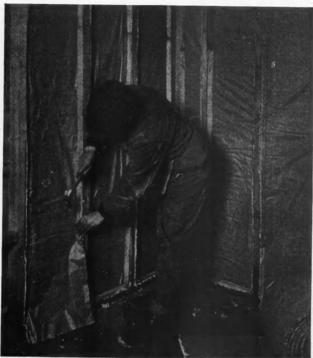
The Insulation Here Shown Is a Wood Fibre Quilted Between Sheets of Special Paper and Is Being Nailed to the Studs Under Lath Strips. A roll of the material, revealing its fleecy nature, is seen at the right.
