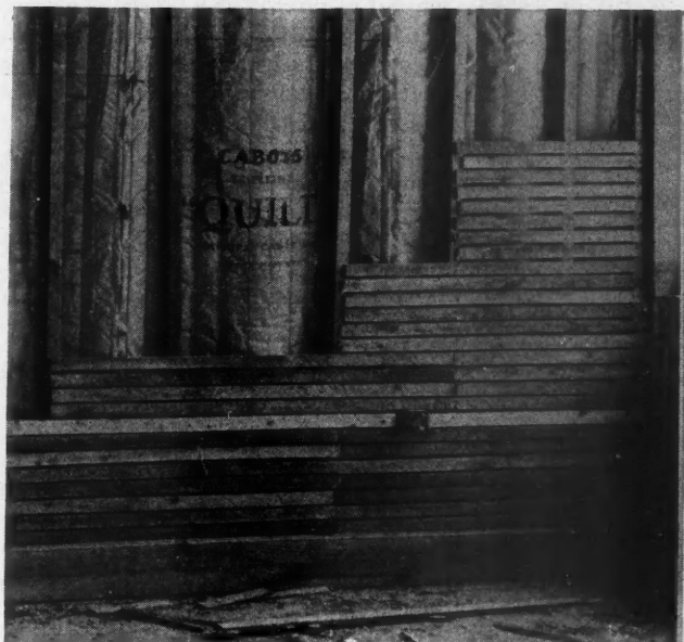
The Insulation Here Shown Between the Studs of a Wall Under Construction Is Made of Marine Grasses Quilted Between Sheets of Waterproof Paper. This insulation is impervious to moisture and has excellent insulating qualities.
