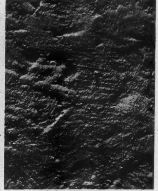
ROUGH CALIFORNIAN A rough cast finish reduced by rubbing with a carpet-covered float
