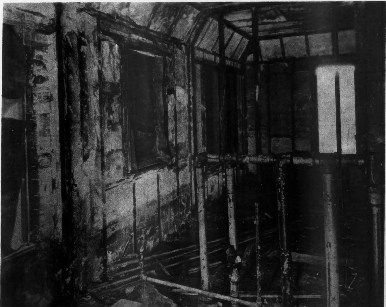
After the Fire—Inside Partitions and Outside Wall Lining Completely Burned; Edges of Studs Charred; Gypsum Insulation, Which Stopped the Fire, Still in Place.
