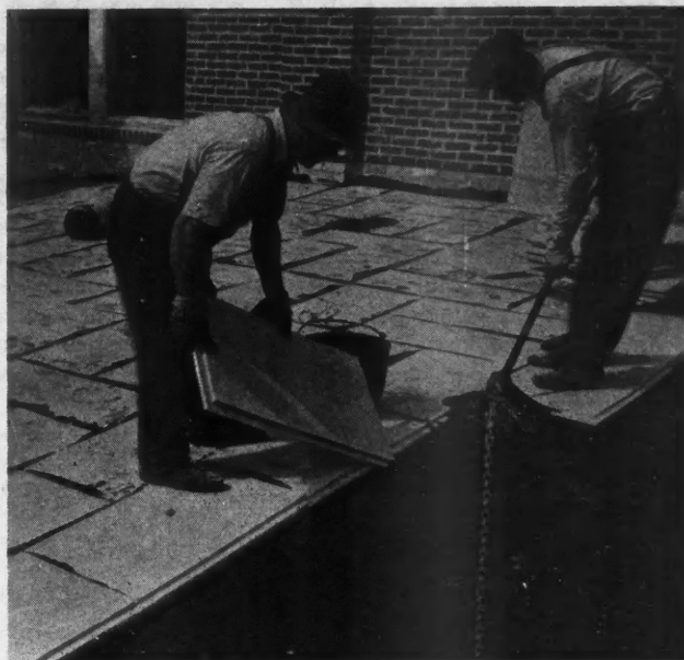
Here We See the Insulation of a Concrete Roof Deck with Sheets of the Pressed Wood Fibre Type. This insulation is mopped over with hot asphalt as a top finish. It prevents excessive heat loss and condensation or drip underneath.
