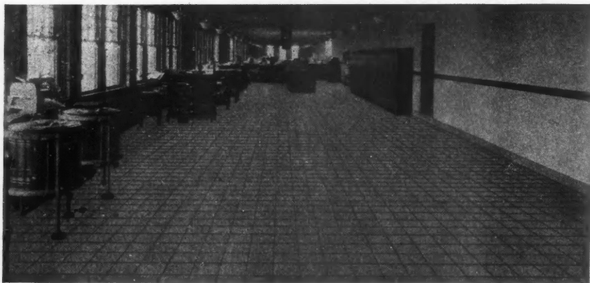
Employers Have Learned the Value of Good Finish, Bright and Clean Surroundings in Factories and Workshops as Well as Offices. Note the well finished, sanitary appearance of this plastic magnesia flooring laid in tile pattern.
