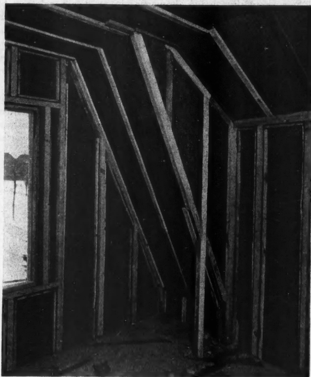
The Insulation Used Between the Studs in This Picture Is Made from Flax Fibres Felted and Pressed into Semi-Rigid Sheets. It has good heat resisting qualities and is non-inflammable.
