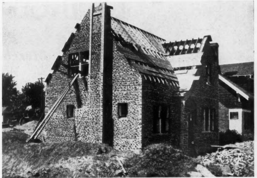
One of the First Houses Built by the Formless Concrete Construction Company, of St. Paul, Minn., Which Is Developing This Novel System.
