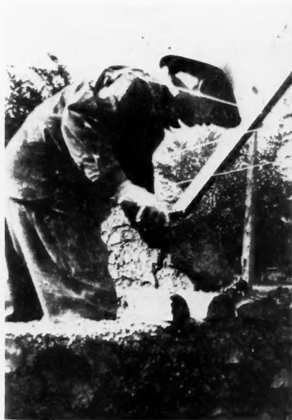
The Wood Blocks Are Laid Up with Cement Mortar Much as Bricks Are.
