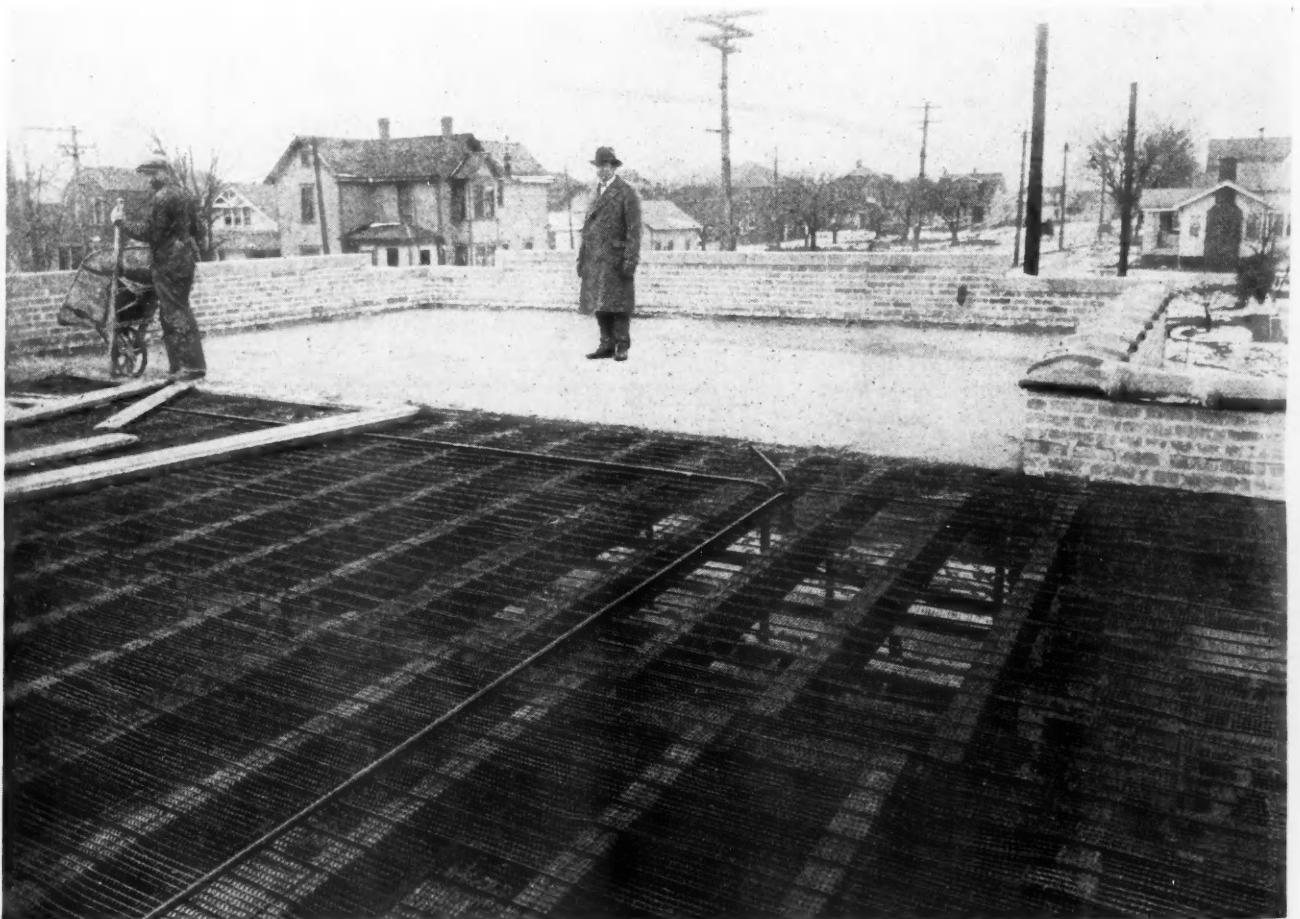
Pouring a Structural Gypsum Concrete Roof, Over Ribbed Metal Lath, at Waukegan, Illinois. Note the handling of electrical conduits and the fact that the roof will support the weight of a man almost immediately after it has been poured.
