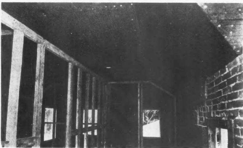
Another Insulating Coat of Corkboard, on Tile Wall and Second Floor Ceiling of a Residence, Which Saves Coal.
