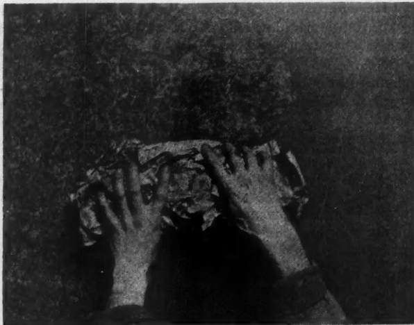
Mottling with Crumpled Paper Is One of the Easiest as Well as Most Effective Techniques to Obtain on Painted Walls. The paper is held in both hands and rolled over and over down the wall.
