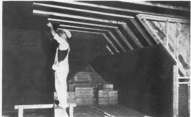
Applying Corkboard Insulation to the Under Side of the Roof Prevents an Appreciable Amount of Heat Loss and Makes Consequent Reduction of Heating Expense.
