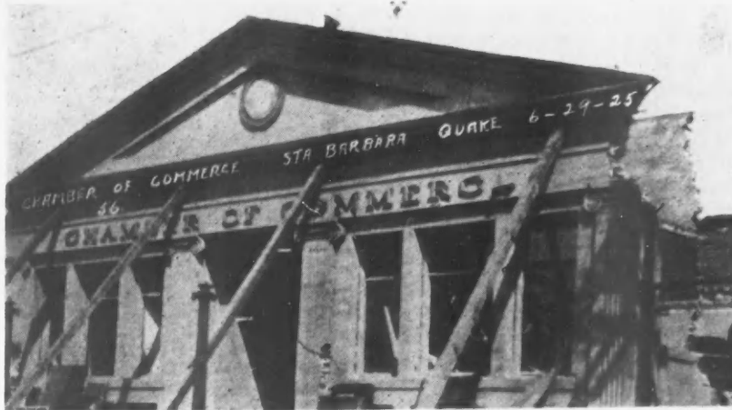
Temporary Bracing to Prevent a Heavy Cornice from Falling Into the Street. Cornices of this sort are dangerous in quake regions.
