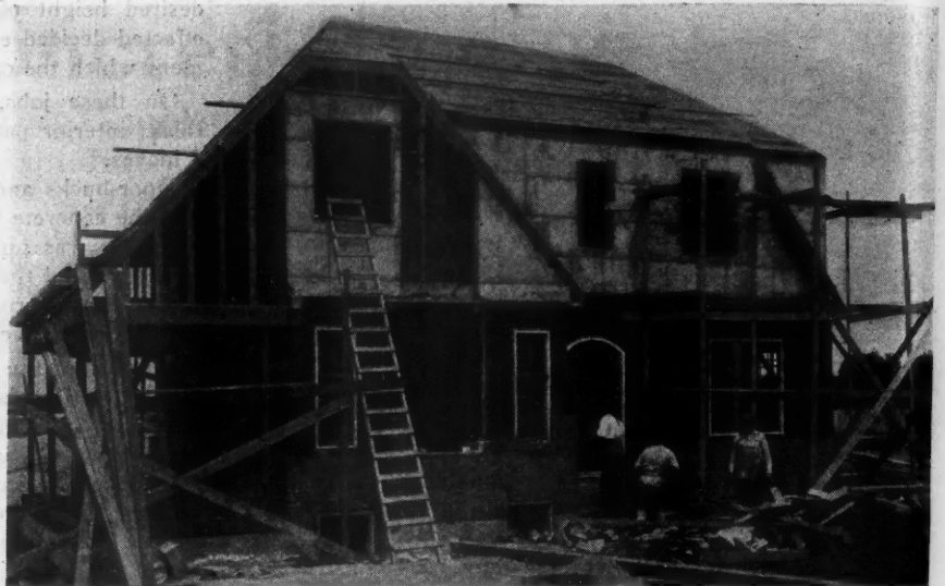
House of Structural-Gypsum Concrete as It Appears When the Walls Are Entirely Poured, the Roof Erected and the Application of the Exterior Facing and Trim Is getting Under Way. In this case, a wooden roof was used, its surface covered with asphalt roofing. The big space in the center has been left open for the chimney. The black color of the lower half of the building is due to the waterproofing compound which, at this time, had not been applied over the entire structure.
