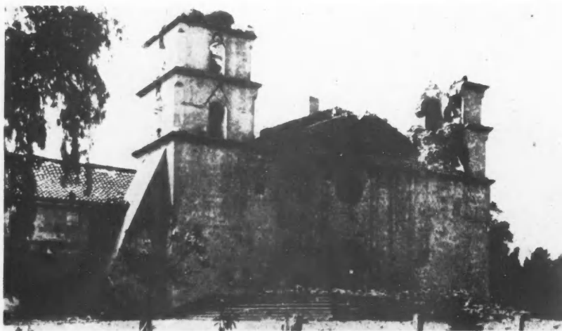
The Heavy Adobe Walls of the Old Santa Barbara Mission Made This Building More or Less Rigid and Only the Towers Were Wrecked by the Quake.
