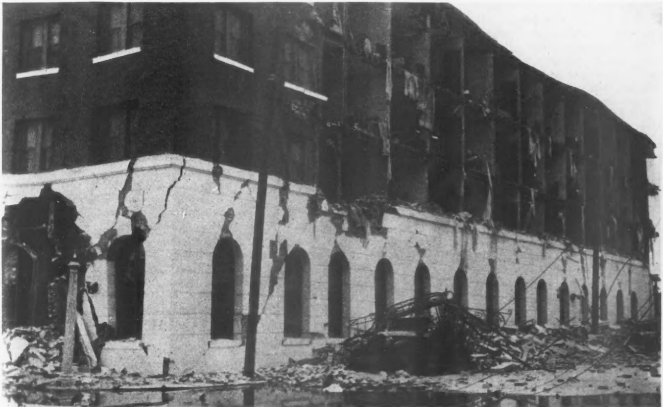
Effect of the Earthquake on a Three-Story Hotel Building Where no Brick or Tile Cross-Partitions Protected the Structure Against Side Thrust.
