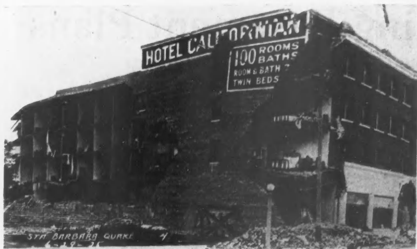
This Shows How Brickwork Sheared Away and Lack of Cross-Partitions and Brace-Rods Allowed the Building to Literally Pull to Pieces. The offset in the word "California" indicates the extent of the sway.
