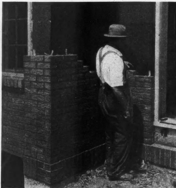
Applying the Brick Veneer for the Exterior Finish Over Walls of Structural Gypsum Concrete. The metal ties are nailed right onto the walls and are embedded in the mortar between the brick courses. Note how tight the concrete sets up against the window and door frames.
