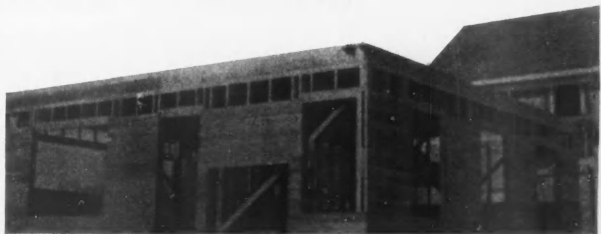
Photo 3—Here Is an Example of 7-Foot 11½-Inch Studs and Short Length Sheathing.
