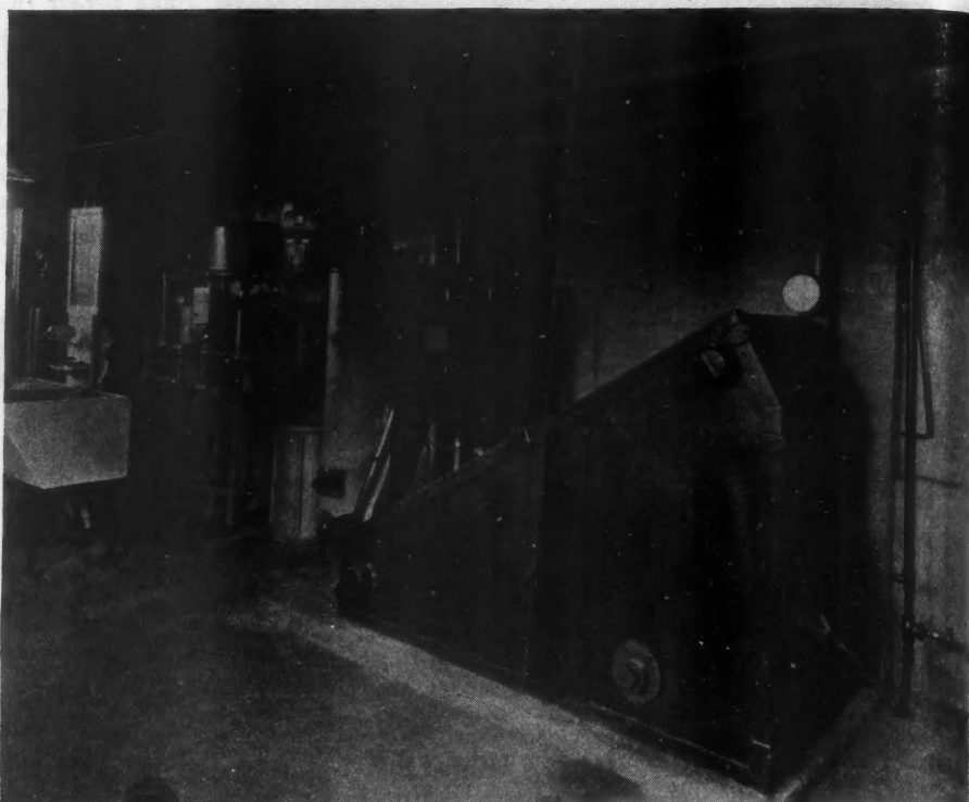
This Picture Shows the Basement of a Bungalow Equipped with a Hot Water Heating Boiler of Triangular Shape Fired by a Motor Driven Oil Burner. This view also shows the water softening apparatus, the laundry tubs and the insulated domestic water heater and storage, gas fired and automatically controlled.
