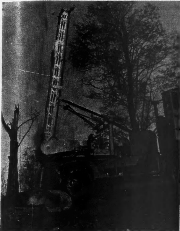
Here Is a View of the Auger at Work Boring Through Solid Rock, an Application Which Is New but Wholly Successful.
