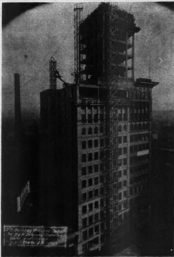
At Dayton, Ohio, the U. B. Building Is 21 Stories, 276 Feet High and Engineers Say the Limit in Height for Reinforced Concrete Buildings Has Not Been Reached.
