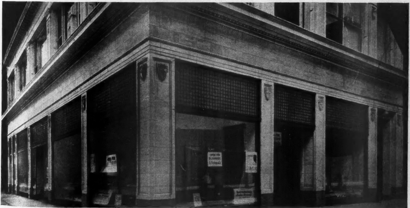
Another Fine Example of a Remodeled Store Front. This is the store of A. Bishop & Company, hats and furs, Chicago. Fine masonry, metal store fronts, the extensive use of prism glass transom lights and fine plate glass windows combine to produce the desired modern effect.
