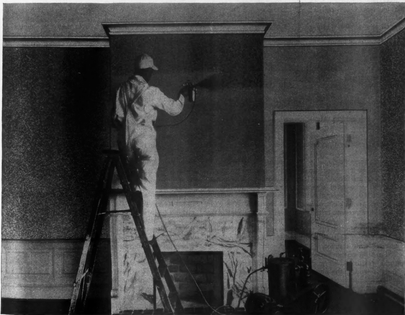
Color Misting, Done with Mechanical Painting Equipment Operated at Low Pressure, Is a New Method of Interior Decoration for Walls. Note solid color of first coated portions of walls. Because of the wide variety of available colors this system of decoration possesses many interesting possibilities.
