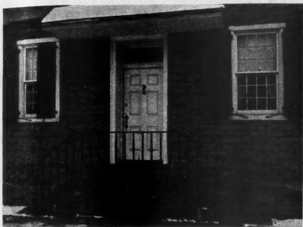
Fig. 3. This Door Is Fitted with a Latch with the Handle on the Outside. The small plate above covers a modern key cylinder. Strap hinges and lag pins can be seen on the shutters. Long iron hooks fastened to the sills hold the shutters open. Mud scrapers are formed in the iron hand rail at the bottom step on each side.
