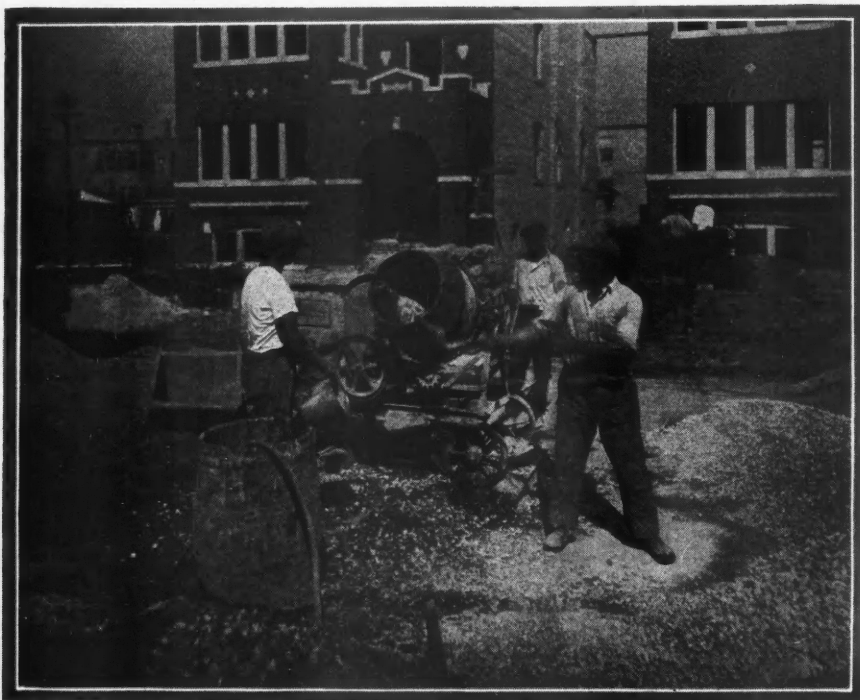
The Materials for This Residential Job Are Being Delivered by Motor Trucks and a Small Tilter Mixer Is Mixing the Concrete for the Foundations.
