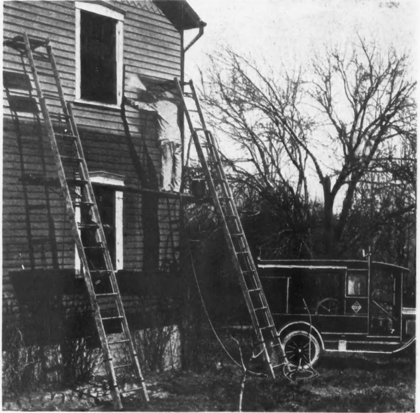
By the Mechanical Method, It Is a Matter of Minutes to Paint the Side of a House and There Is a Big Saving in Cost.
