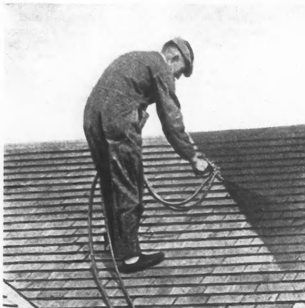
Large Roof Areas Can Be Quickly, Economically and Thoroughly Painted with Mechanical Equipment and Their Life Is Greatly Increased by Paint.
