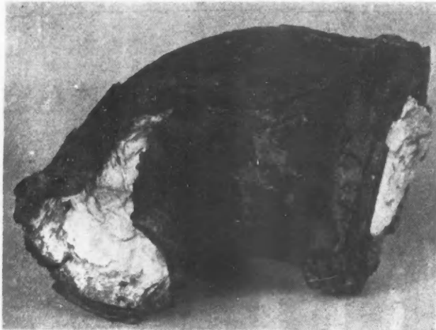
What Hard Water Does in a Few Years to the Water-back in the Furnace. This photo, actual size, was taken of a pipe removed in Indiana.
