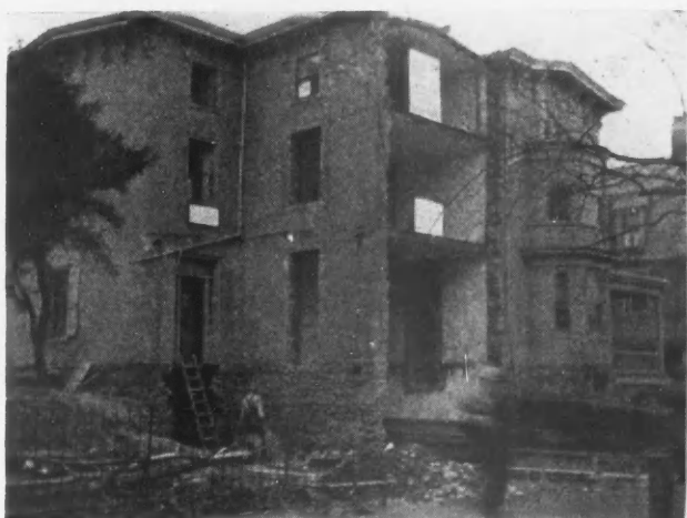
An Old Three-Story House in the Process of Being Made Over Into Stores and Apartments.
