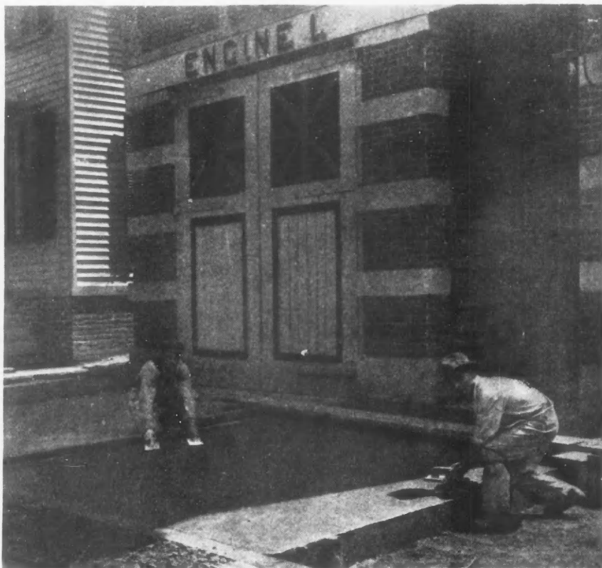
Obviously the Pavement in Front of the Firehouse Is One That Should Not Be Out of Service Long. This one at Somerville, N. J., was hard enough for use in 24 hours through using quick hardening cement. It was reported to have been as strong at 24 hours as Portland cement would have been at 28 days.
