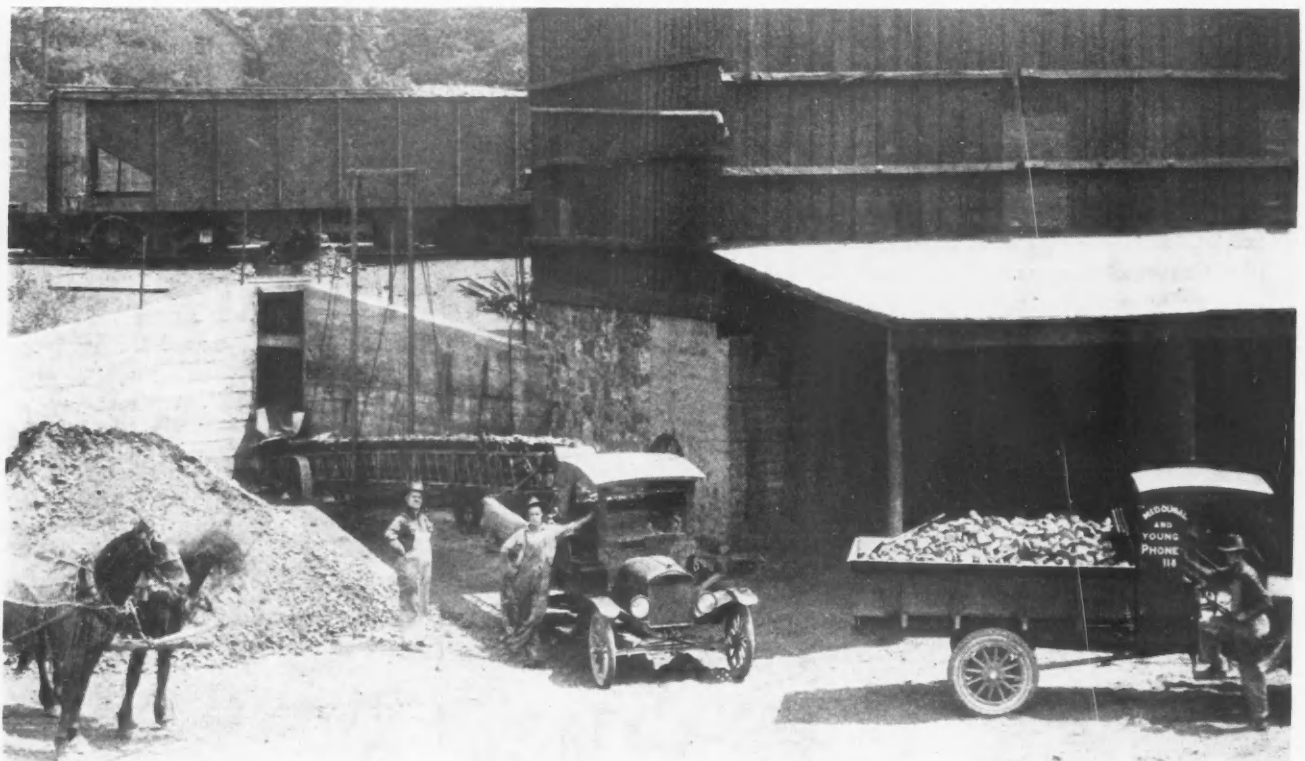
Here Is a Fine Example of the Quick Transfer of Bulk Material Direct from the Railroad Car to the Job by Means of a Power Loader and Light Trucks. With such an equipment there need be no delays, no tying up of needed cars by slow unloading methods and no expensive handling.
