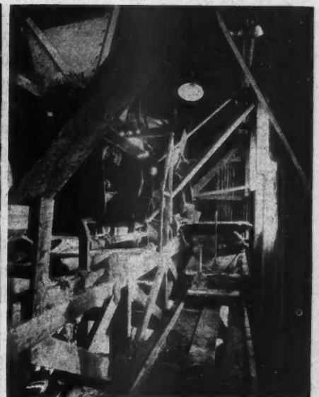
Fig. 4. The Discharge End of the Mixer with Electrically Driven Car Which Distributes the Concrete into the Bins Which Feed the Brick Machines.
