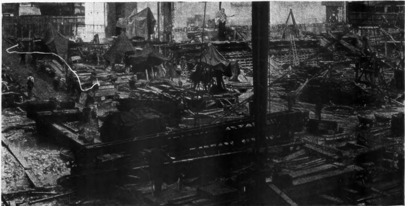
Single Electric Caisson Winches Were Utilized for the Gigantic Task of Digging the Caissons for the New Palmer House, Chicago, Which Will Be the Largest Hotel in the World. The winches are shown under the canvases in the picture. Above is a closeup view of one of the winches.
