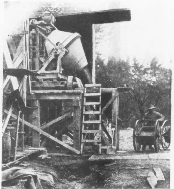
Close-Up View of the Tilting Mixer Discharging. The Power Loader and Extended Track Make It Possible to Take the Aggregate from the Lower Level to the Hopper Above.
