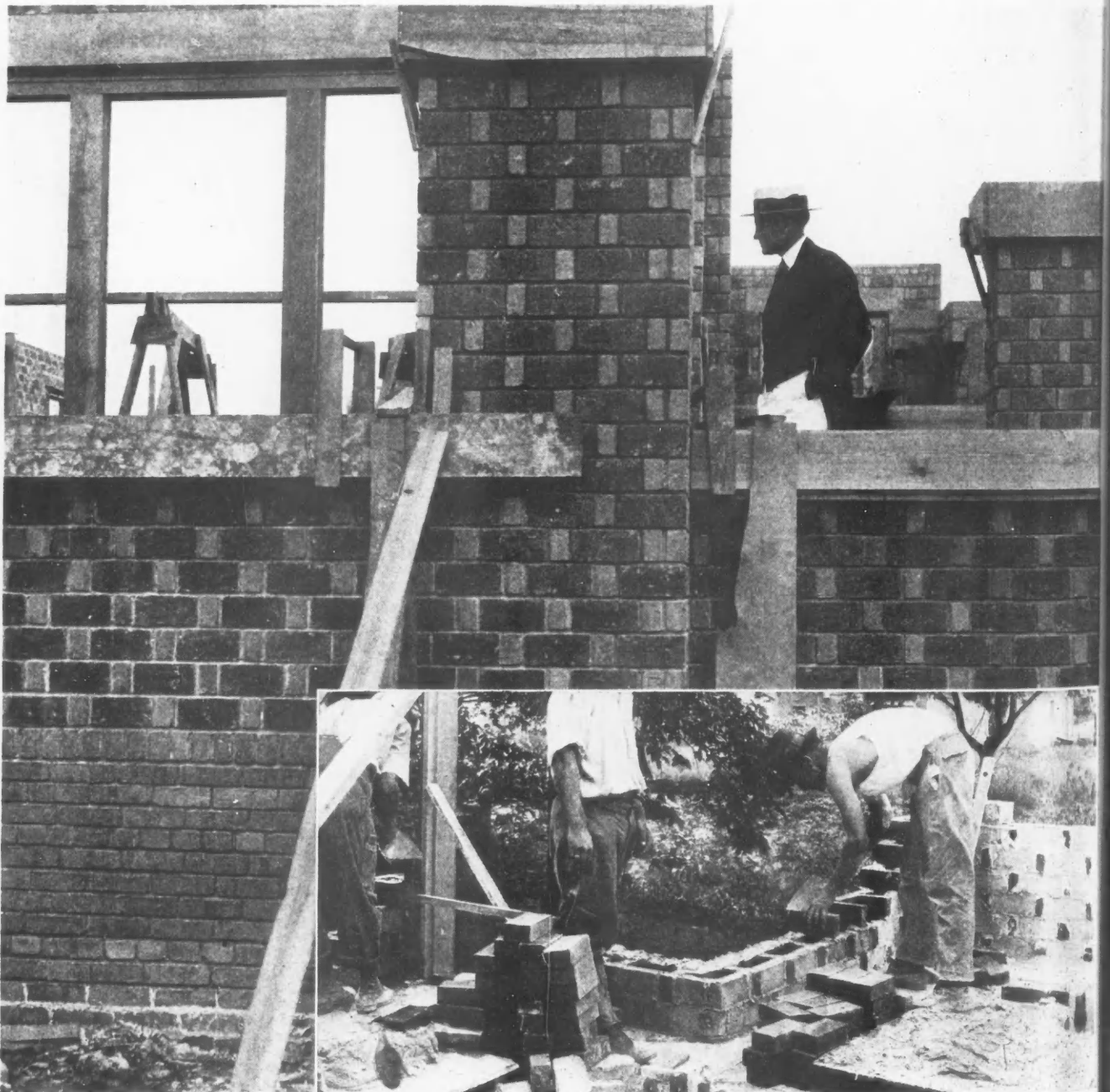
Ideal Walls Under Construction. Note Pleasing Appearance of Rough or Wire Cut Surface of Stretchers in Combination with Smooth Headers.
