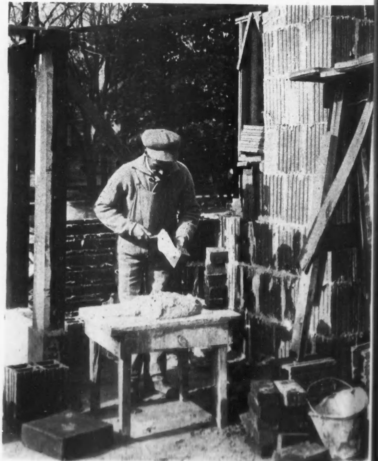
The Mason's Trowel and the Carpenter's Hammer Are Busy Tools in These Active Building Days.
