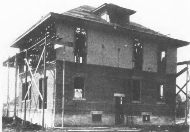
Second Story Finish with Waterproof Fibre Board and Panel Strips Will Present the English Half Timber Effect.
