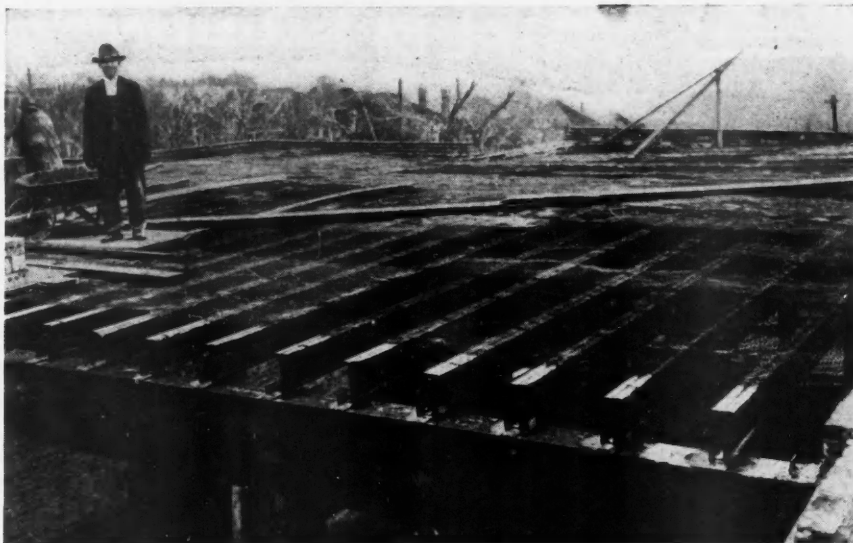
Steel Joists Supported on Top of I-Beam with Metal Lath in Place for Thin Concrete Floor Slab.
