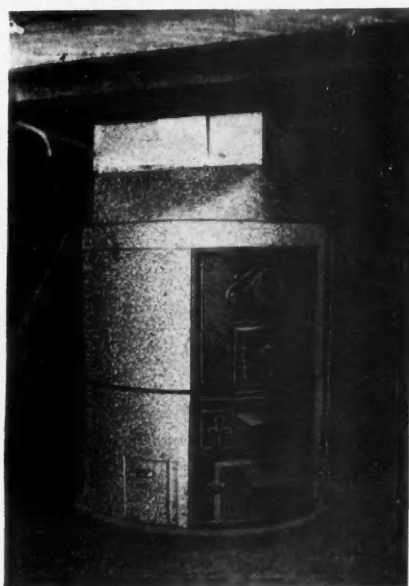
Furnace Installed in Basement. The Heat Is Regulated by the Chain Arrangement Which Is Operated from Upstairs.
