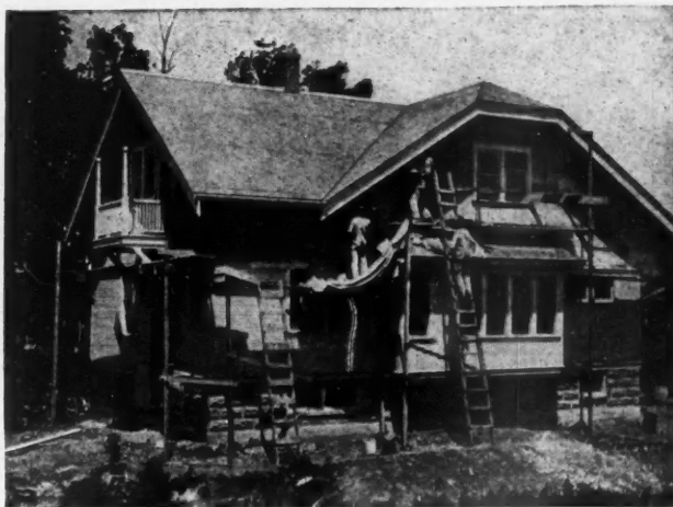
Putting Stucco on New Parsonage at West Allis, Wis. It Is Frame and Stucco.
