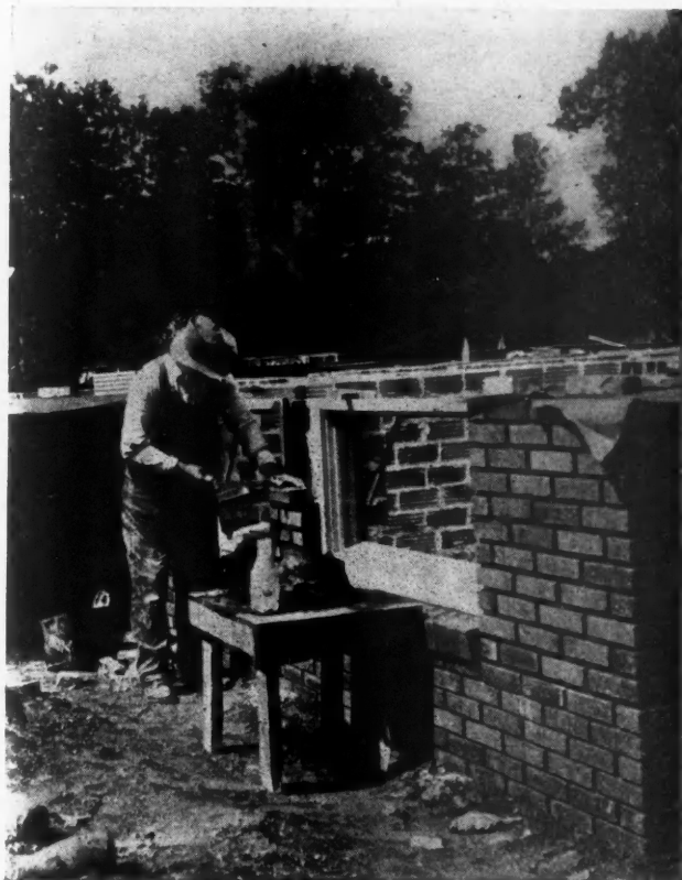
Raking Joints in a New Brick Job. This Joint is Very Attractive and is Used in Fancy Face Finishes.
