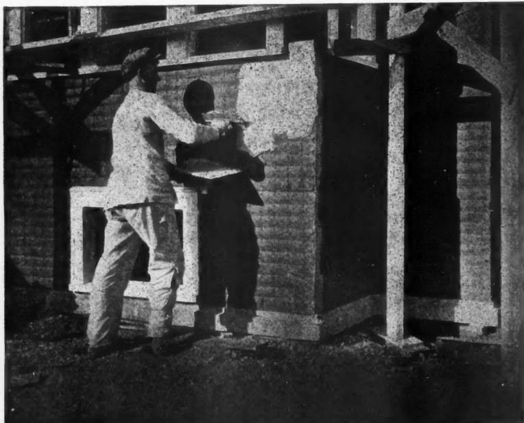
Applying Stucco to Special Fabric Backing which is Fastened Directly to Studs Without Sheathing.
