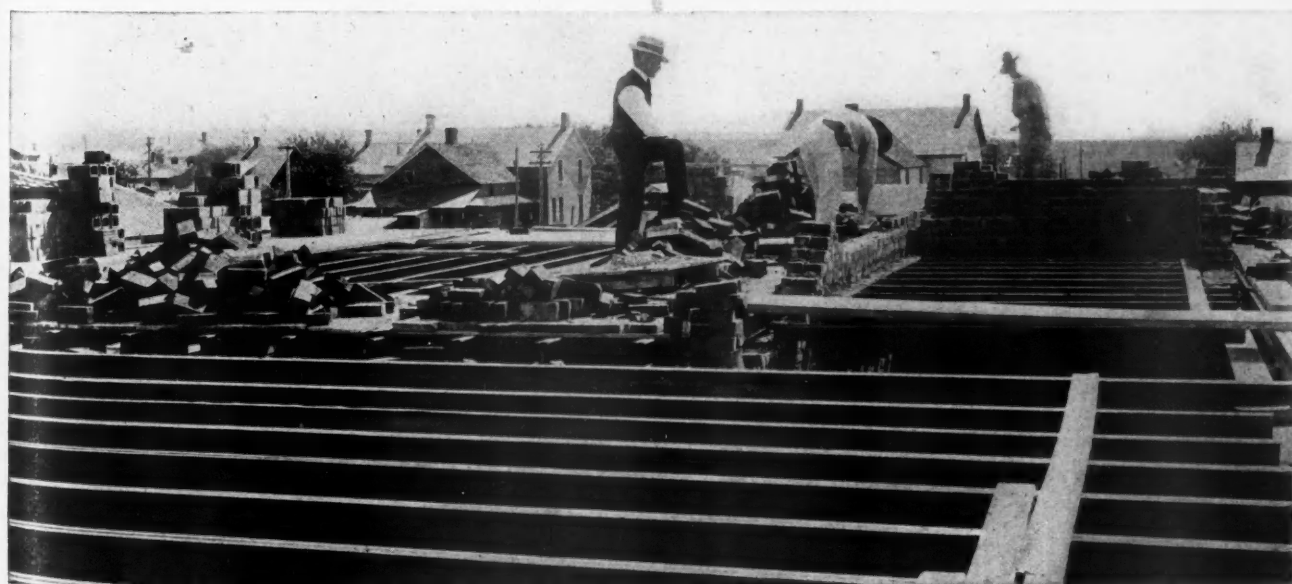
Steel Lumber Joists Were Used In This High School Building at Sidney, Neb. They Are Supported on Brick Bearing Walls.
