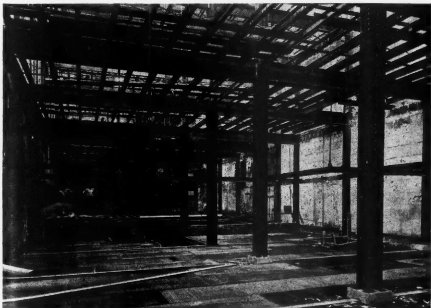
Telephone Exchange Building, Akron, Ohio. This Building Had Been Guttled by Fire. It Is Being Reconstructed with Structural Steel and Steel Lumber Joists.
