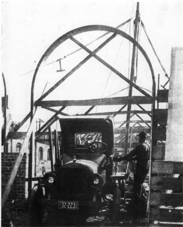
Frank P. Pursell, Building Contractor in Los Angeles, Has Effected a Great Saving on His Truck by Adding a Winch for Lifting Girders into Place in a New Building. It Is Driven Off the Truck's Countershaft.
