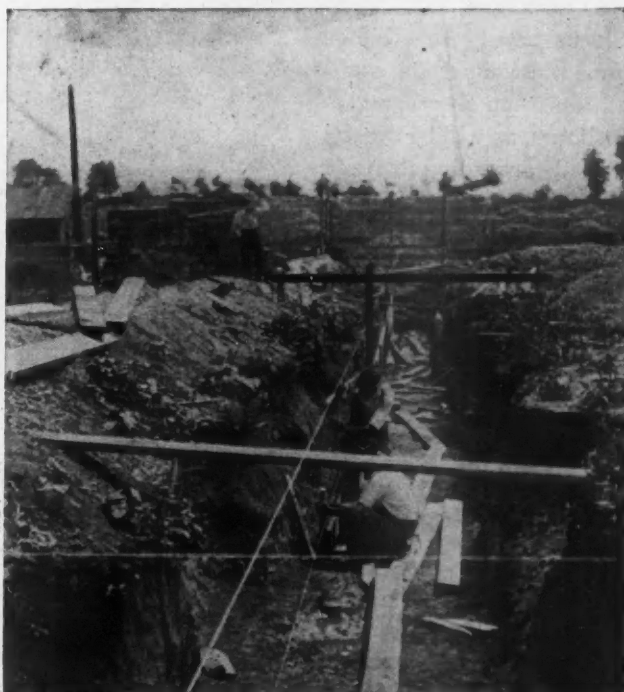
Fig. 6. Erecting the Forms for a Foundation Footing. The Footing Is of Concrete Deposited in Place, and in Residence and Other Small and Moderate Building Construction Is Usually Made 12 Inches Deep and 16 to 24 Inches in width, Depending on Soil Conditions.
