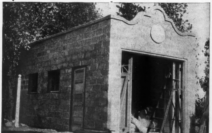
Concrete Block Ready for Stucco Coat. The Roof Is Supported on 2 by 10 Joists Which Extend Crosswise at a Height of 9 Feet Above the Floor. The Stucco Is Applied Direct to These Blocks, Which Make a Good Bond Because of Their Rough Texture.
