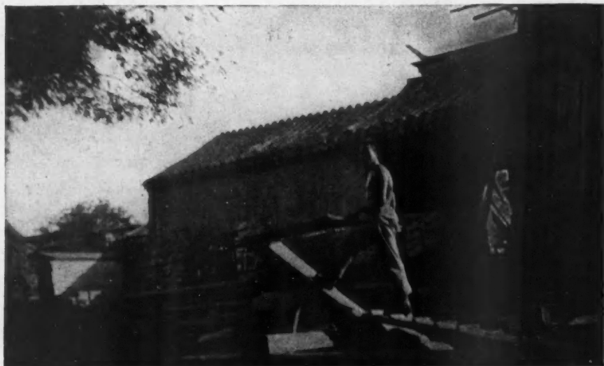
The Chinese Carpenters Whipsaw the Timbers to the Proper Dimensions on the Job, Using Crude, Heavy Saws. This Photograph Was Taken in Peking, and Shows a Carpenter at Work with the Heavy Saw, Shaped Much Like a Rifle.
