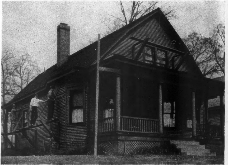
Before. Frame House in Springfield, Ill., Being Prepared for an Overcoating of Stucco. It Was Beginning to Look the Worse for Wear.
