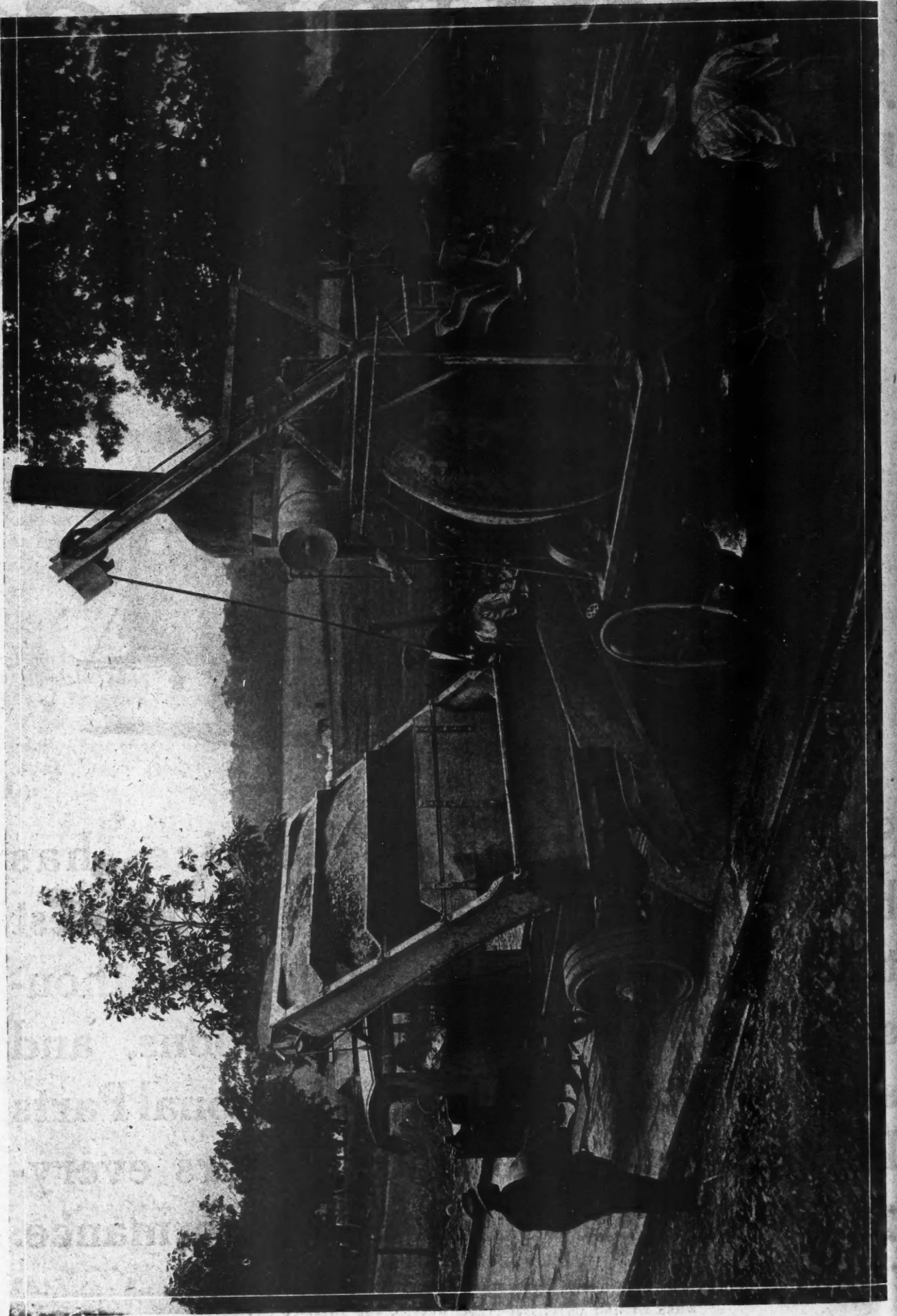
The Contractor Who Owns This "Service" Truck Has Devised a Unique Labor-Saving Device for the Body of His Truck. Each of the Four Compartments Contains Enough Gravel or Crushed Stone and Sand to Fill the Skip in the Mixer. As the Dump Body Is Lifted, Each Section in Turn is Released and Dumped.
