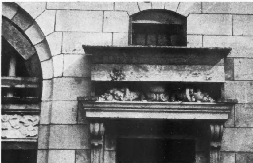
Protection of Concrete Architectural Stone, and in Fact All Protruding and Exposed Part of the Surface While Construction Is in Progress, Is Very Important. Rough Box Protection, Like That Shown, Is Inexpensive.
