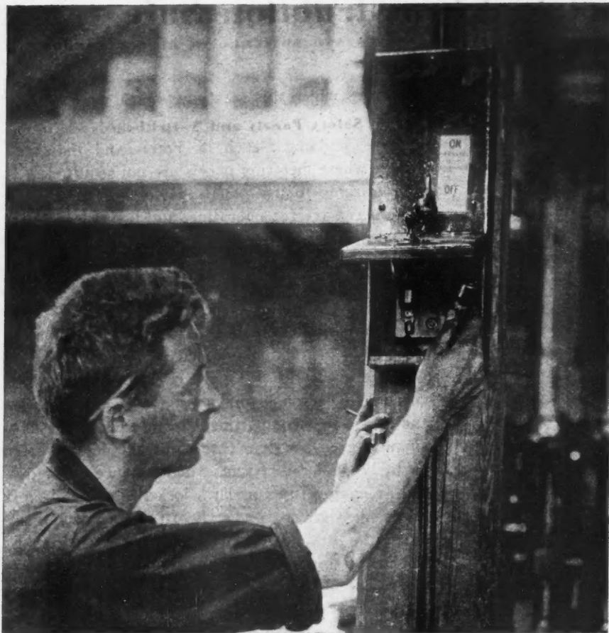
This Fuse Compartment Cannot Be Opened Unless Switch Is in the Off Position Because of the Safety Arrangement in the Switch. Safe Electrical Construction of This Type Is Being Installed in Shops and Factories to Protect Employees.
