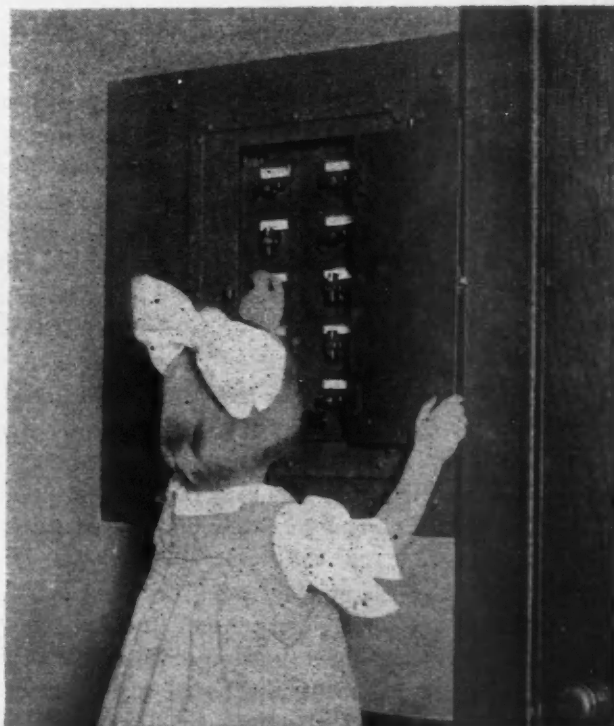
Making Electrical Construction Safe for the Children. The Safety Panel Installed in This Home Reduces the Risk Connected with Switches.
