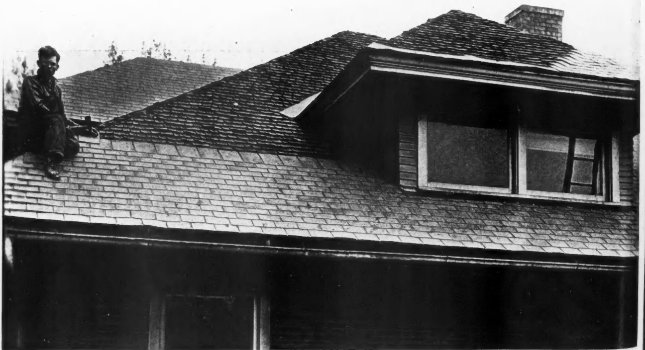
Re-roofing Over the Old Shingles. Purnell Bros., Oak Park, Ill., Put the New Roof Material Right Over the Old, and Claim a Great Saving in Cost. No Labor Is Required to Remove the Old Shingles, Neither Does the House Owner Have to Clean Up the Litter.
