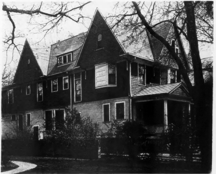
Showing the House After the New Roof Is On. None of the Old Shingles Was Removed, But the Job Was First Class, as Will Be Seen by the Picture.
