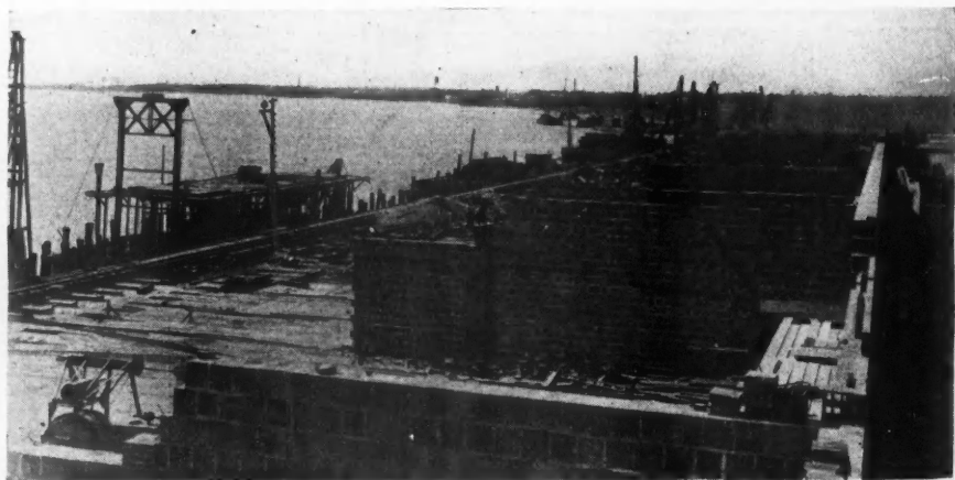
Fig. 6. View Showing Construction of Storage Building at the Great Charleston, S. C., Port Terminal. The construction of dividing fire walls is clearly shown.
