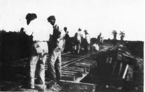
Movie of F. Hutson's Bridge Moving Job. The Top Picture Shows the Bridge Being Placed on the Railroad Tracks; the Center Picture Shows It Being Taken to Its Destination, and the Bottom Picture Shows the Bridge in Place. The Bridge Was Moved a Mile and a Half in Seventeen Minutes.
