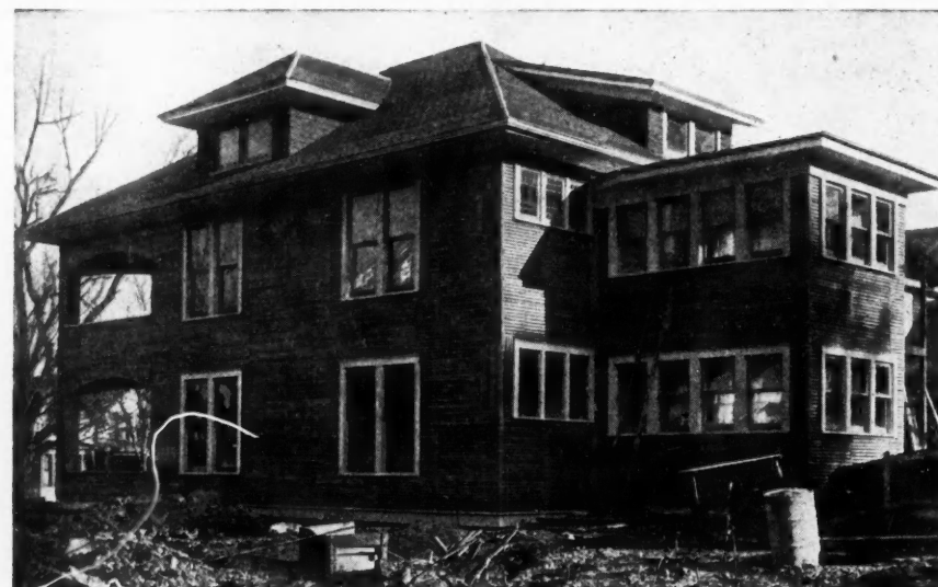
Old House Being Remodeled Into a Two-Flat Building; Stucco Board Ready for Plastering.
