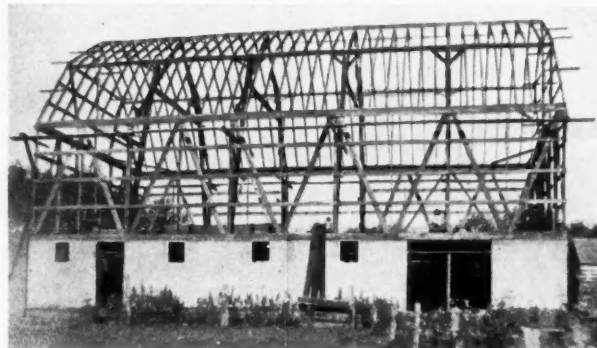
Construction View of Plank Frame Barn Built on Farm of Frank Lowe, Near Fairmont, Minn., by George Hengel.
