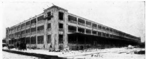
New Reinforced Concrete Structure Which Houses the Flint, Mich., Assembling Plant of the Chevrolet Motor Company.
