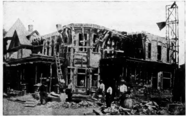
Work in Progress on the Residence Designed and Built by Ralph C. Bennett, Indiana, Pa. Carpenter Work Done by Morris A Wolf.
