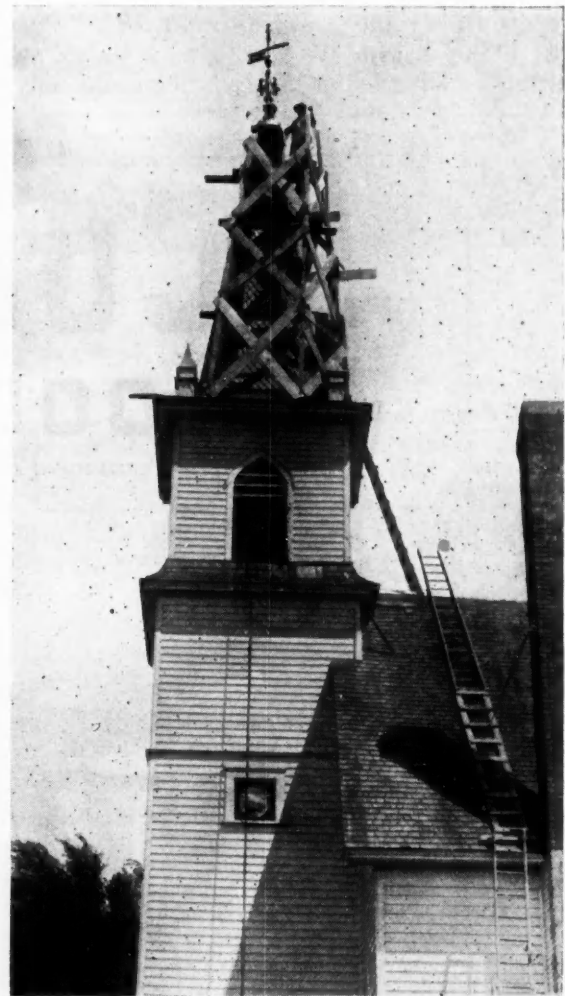
Repairing the Damage Done by Lightning. Work Being Done by P. C. Paulson, of Madelia, Minn.
