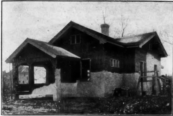
RIB LATH Residence of H. A. Ertz, St. Paul, Minn., during construction.
