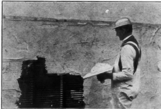
Note perfect clinch of plaster on RIB LATH, with no dropping off.
