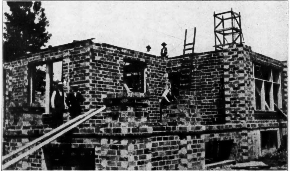
Laying up Davenport Vitrified Building Blocks, to Be Finished Later with Stucco
