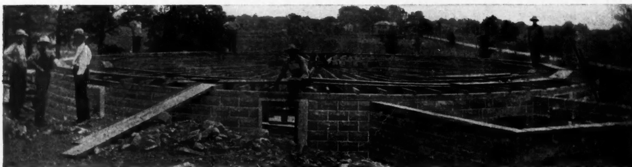
Foundation is Cement Blocks—Round Barn Built by O. H. Bordner, Orland, Ind.
