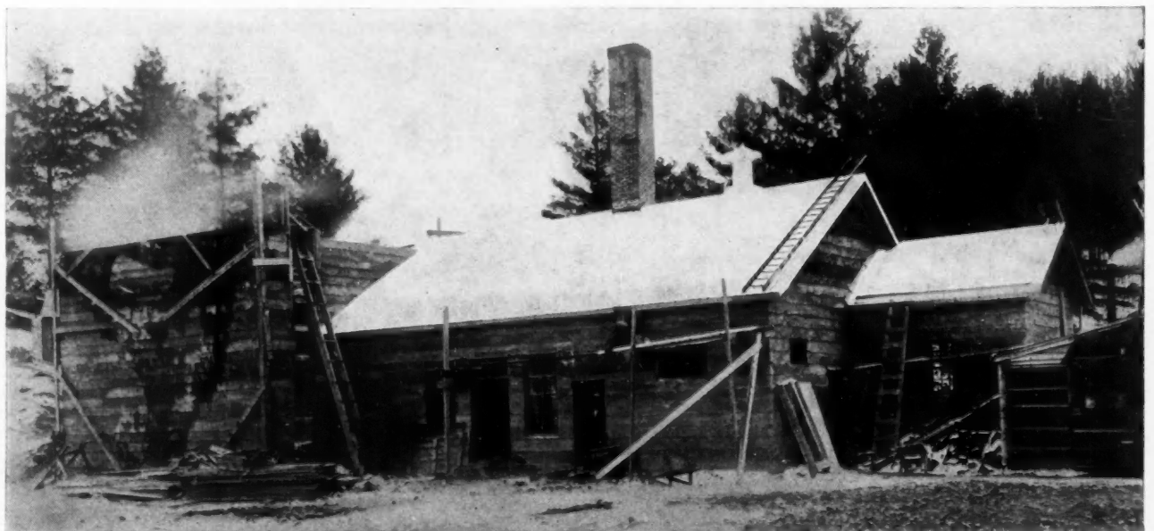
Thin Double Concrete Walls Laid and Steam Cured in Freezing Weather at Wells River Junction, Vt.
