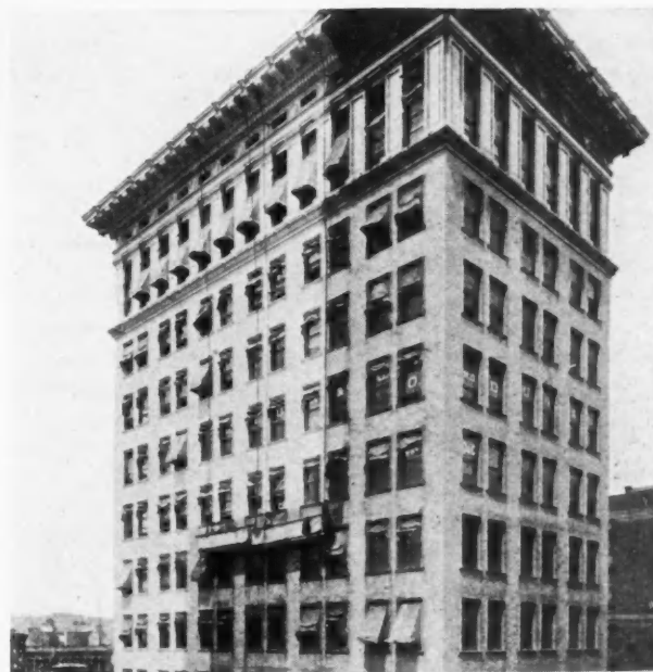
Workmen on Hanging Scaffold "Shampooing" the Ingalls Building, Cincinnati, Ohio, at About the 12th Floor
