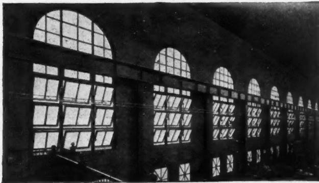
Pond Operating Device in Dynamo Room, Washington Terminal. 99 Sash in 3 Lines, 600 Lineal Feet Operated with One Gear.
