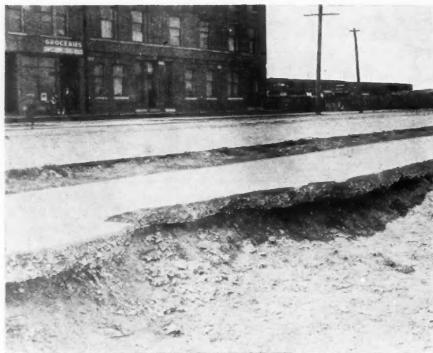
Result of Not Protecting the Edge
