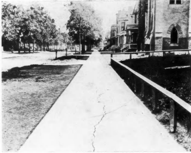
Crack Resulting from Poor Foundation
