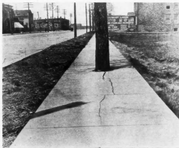
Crack Caused by Tree
