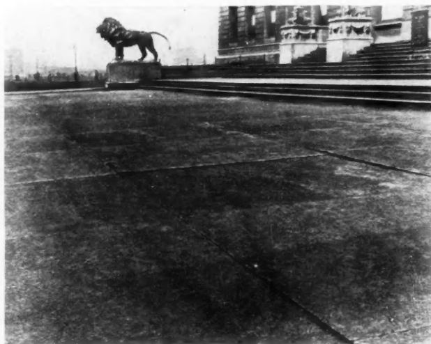
Sand Joints Saved this Walk
