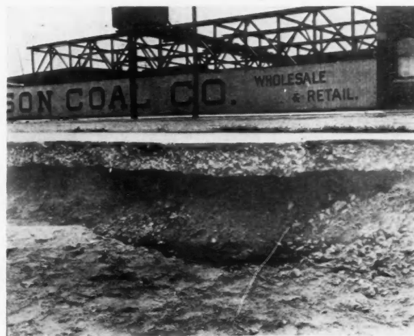
Proper Fill Is Lacking
