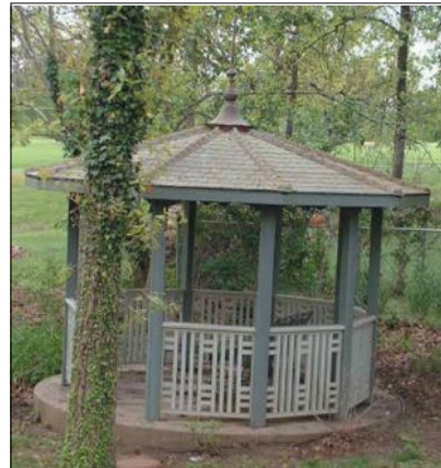
This gazebo features W.F. Norman's Style "A" shingles with its continuous hip finish and a custom-made finial on top.
