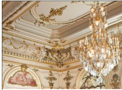
John Canning Studios restored and conserved the ornamental plaster and elaborate murals throughout the Cosmos Club Warne Ballroom in Washington, DC.
