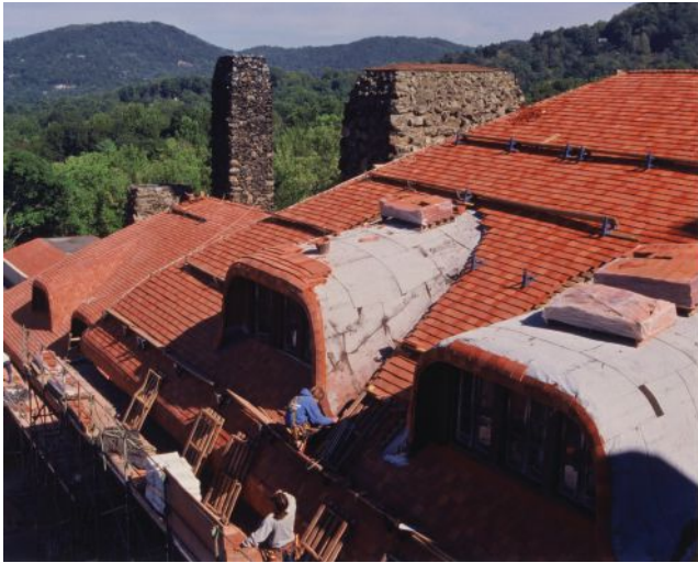
Craftspeople installed the Ludowici multi-hued red clay tile for this roof in Asheville, NC.
