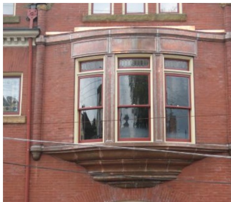
NIKO Contracting Co., Inc. fabricated and installed this custom copper radiused bay window surround.
