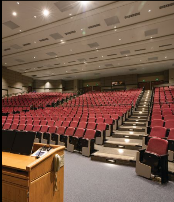
ABOVE LEFT: LED retrofit of existing Rambusch fixtures, installed from below, exceeding previous light levels and cutting energy costs. Penn State University, State College, PA.
