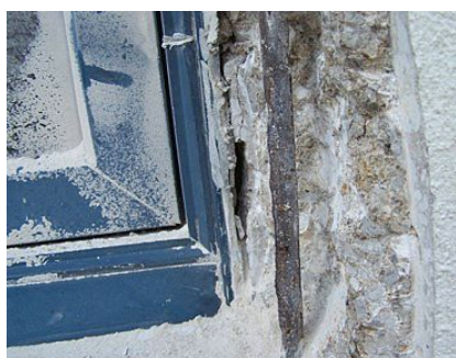
FIGURE 3 Rebar with shallow cover oxidizes, causing concrete to spall
