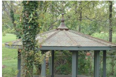
This gazebo features W.F. Norman Corp. 's style A shingles with its continuous hip finish and a custom-made finial on top. Click on No. 520
