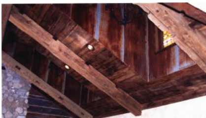
The hand-hewn beams on this ceiling were supplied by Carlson's Barnwood ; the firm also supplied the antique stained glass window and the rusty antique corrugated tin in the dormers.
