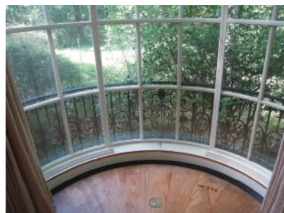
Allied Window supplied the Magnetic One Lite (MOL) "invisible" storm window for an historic building in Dumbarton Oaks, Georgetown. Click on No. 690
