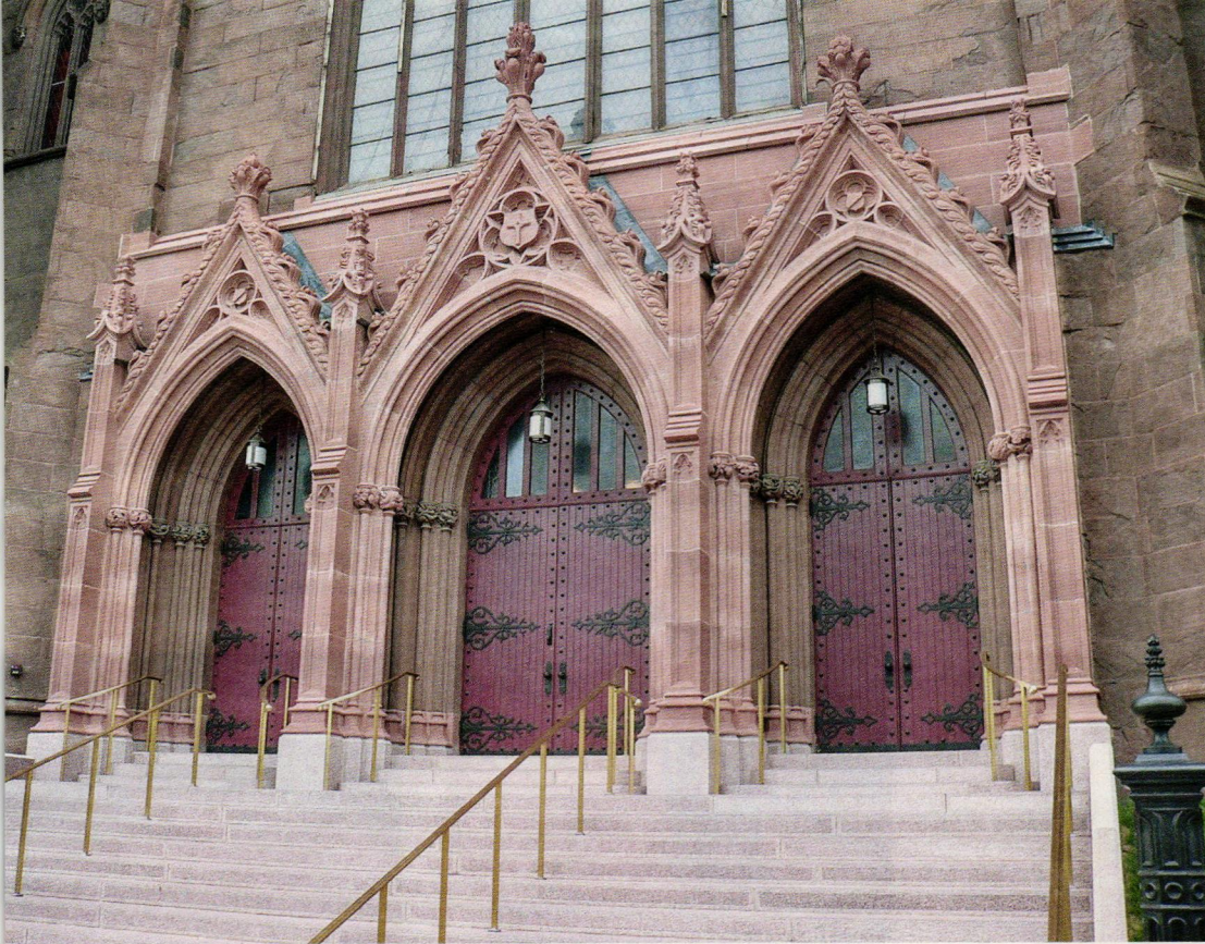
LEFT: Old World Stone fabricated replacement limestone for the restoration of the entry porticos at the Cathedral of the Immaculate Conception, Albany, NY.
