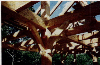
Vermont Timber Frames uses reclaimed and newly cut timbers for its timber-frame structures.
