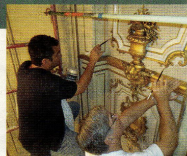
John Canning and David Riccio of Canning Studios are shown here preparing the decorative finishes, conservation and restoration samples for The Cosmos Club, Warne Ballroom in Washington DC (built 1901). Click on no. 5100.
