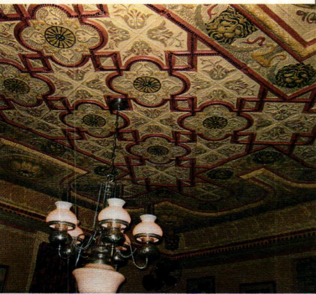
This Oriental-style ceiling was created using pressed-tin panels from W.F. Norman Corp.
