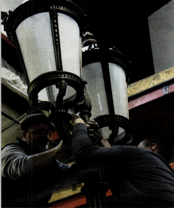
LEFT: Baird helps Jon Varner of Historical Arts & Casting, Inc. install the head of a restored light fixture for the Grand Central Terminal in New York City. Photo: courtesy of Historical Arts & Casting, Inc.
