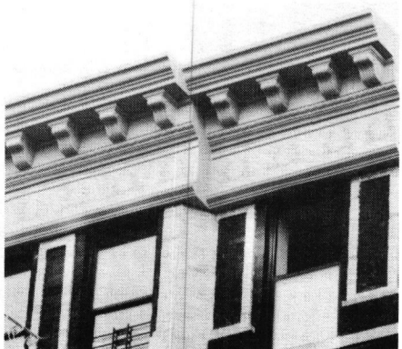
"Stuart Style" FRP cornice, fabricated by ARCHITECTURAL FIBERGLASS CORP. and installed in downtown Manhattan. Write in No. 640
