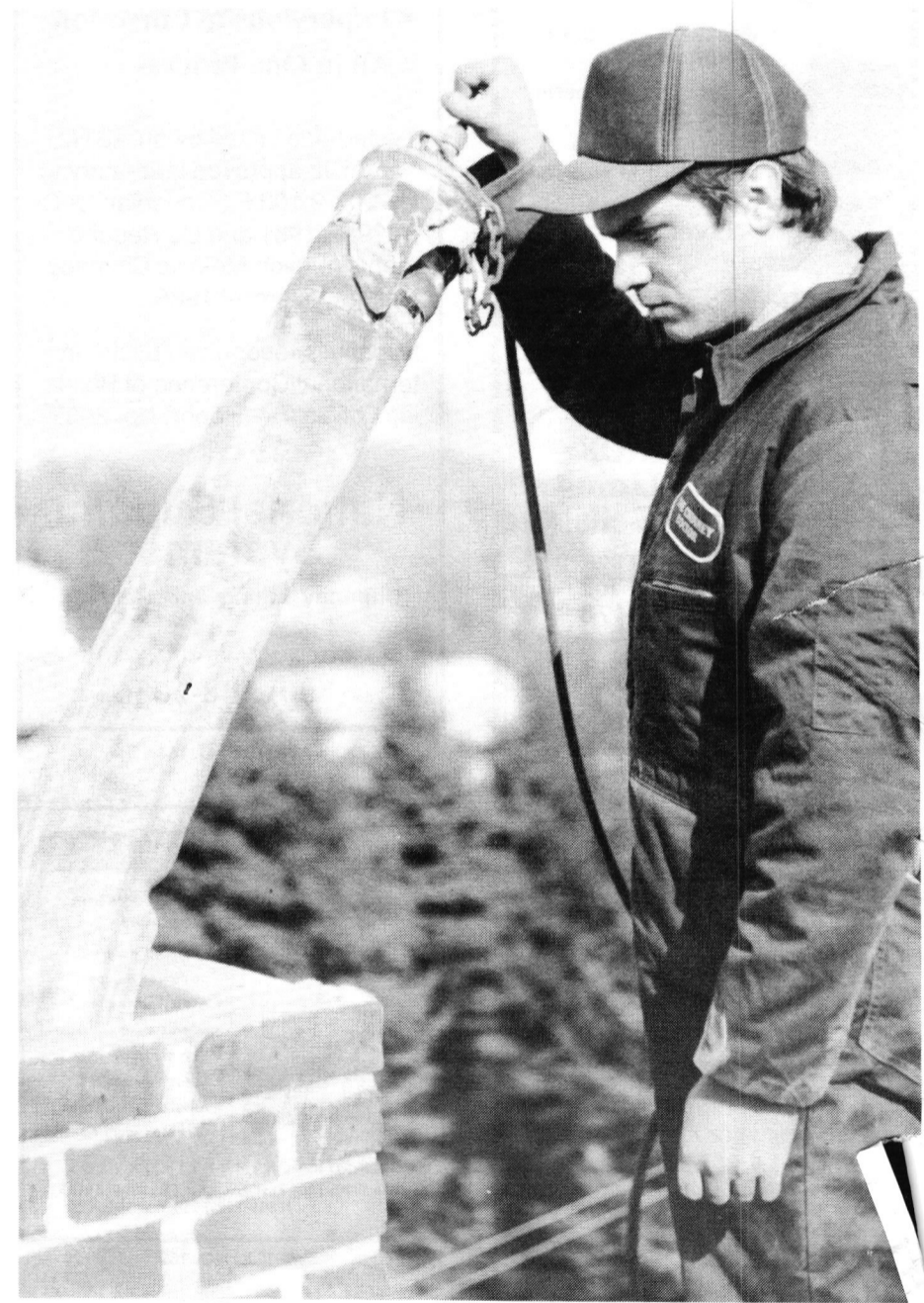
NATIONAL SUPAFU SYSTEMS employee holding the Supaform which has been inflated to the proper flue size. Supafu material is then pumped in around the form. Write in No. 164
