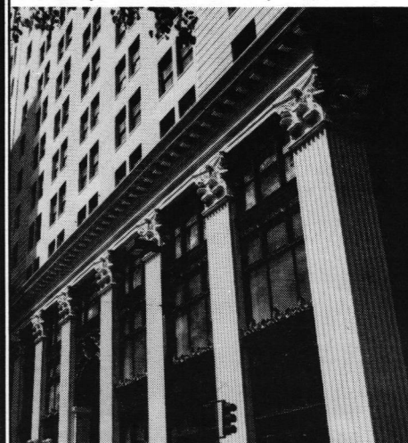
Restored facade of Widener Building. Capitals and horizontal ornamentation were made of fiberglass reinforced polyester resin in Polytek Rubber Molds.
