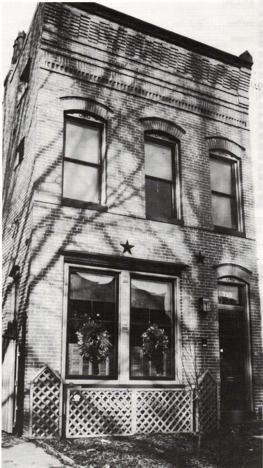
The nearly finished townhouse-office, with trelliswork disguising pipes, rebuilt windows painted original colors, and further sagging controlled inside by tied-together joists.
