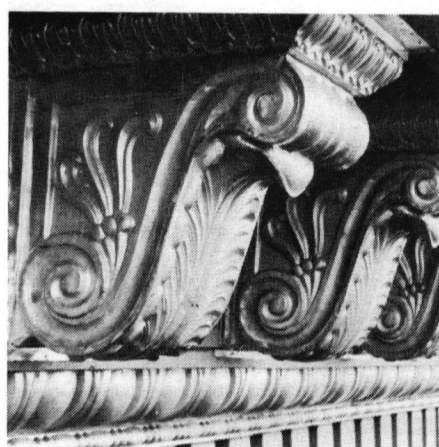
A metal cornice restored at a Manhattan upper east side residence by L.P. KENT Corporation , sheet metal and roofing contractors. Write in No. 441
