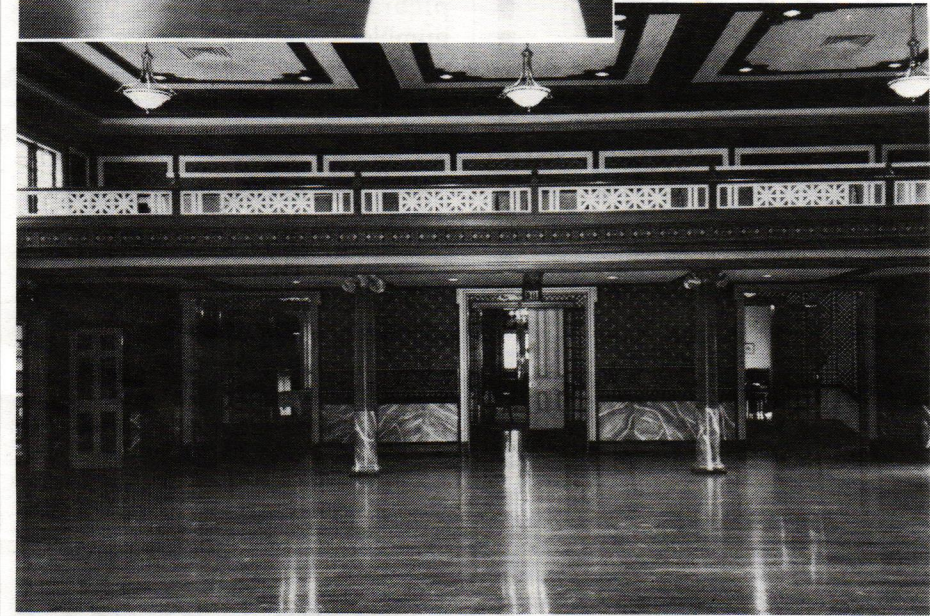
(Top photo - before) In the auditorium, skinny three-inch steel columns supported the balcony; a cornice section had disappeared to make way for a projection booth; unfinished gaps in the balcony railing posed safety hazards; French doors had been painted green, including the panes. (Bottom photo - after) Ionic columns now enclose steel columns; grillwork panels fill railing voids; the cornice has been in-filled; and the French doors are restored to original mahogany color.
