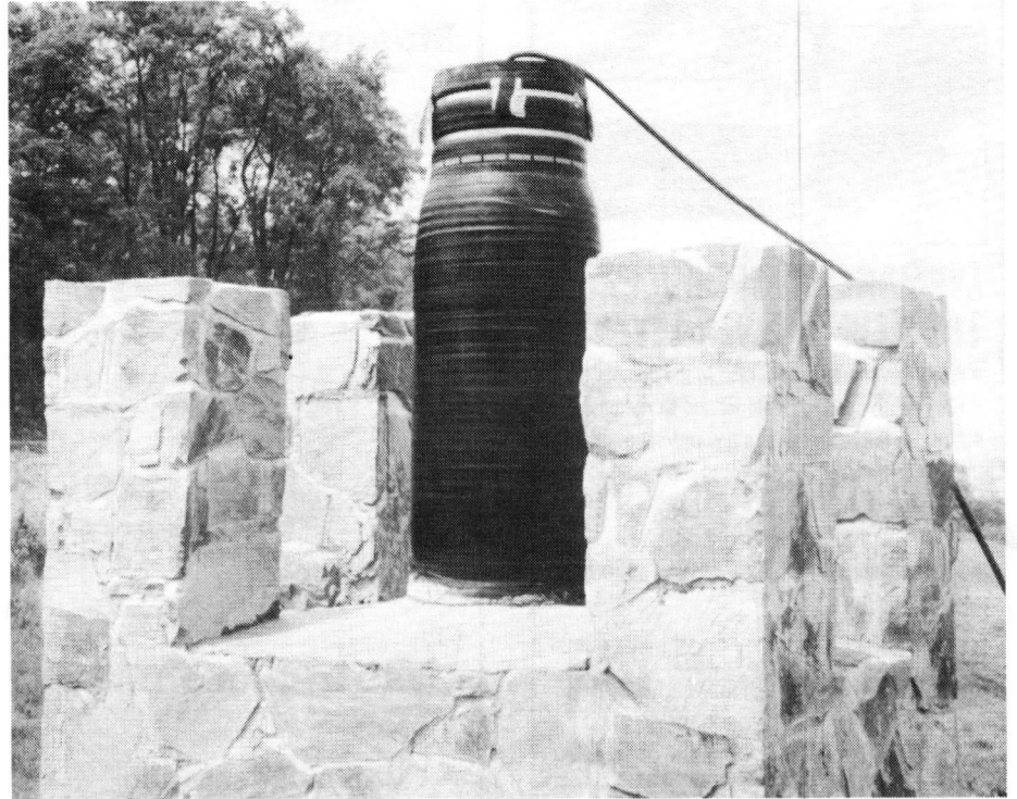
The near-completion of a stove chimney with a cast-in-place liner. As the tube is deflated, it is slid out. GOLDEN FLUE, INC. Write in No. 174
