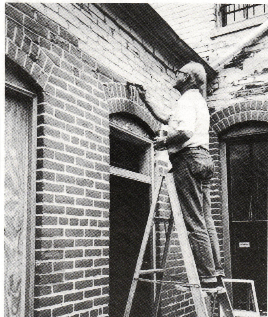
Brown painting bricks on his c.-1885 townhouse-office; the original brick surfaces were hopelessly slathered with tar.
