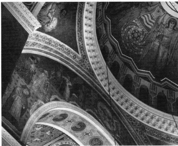
Dome detail: Johnson supervised the restoration of the plaster brackets and borders around windows, as well as the cleaning and touching up of the original paintings on canvas.
