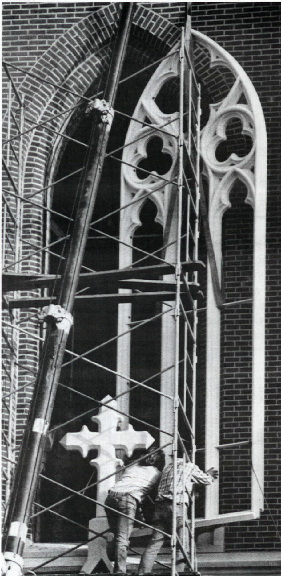
Installation crew from BOVARD STUDIO sets in a new hand-carved mahogany window frame that incorporates a polycarbonate storm window and new stained glass. The storm window channel is built right into the frame. Write in No. 769
