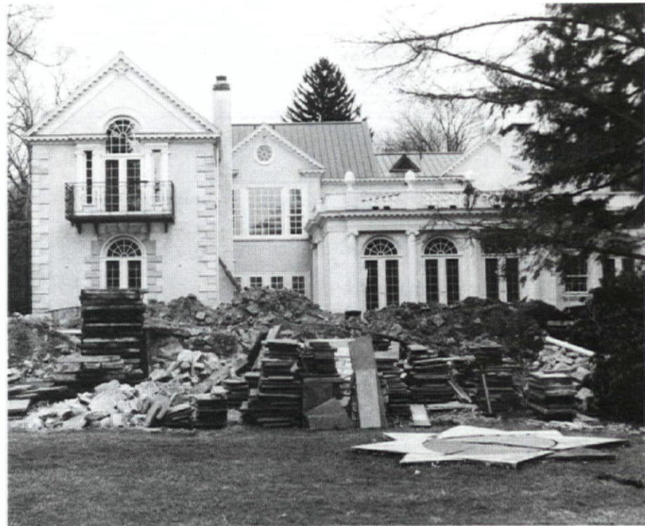
A classical country house under construction. Associates Ann Sutphin AIA and Tami Siegal ASID were in charge
