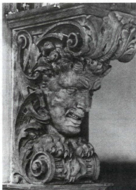
ARCHITECTURAL REFINISHING removed a thick crust of white paint from this corbel at Yale University. Write in No. 724
