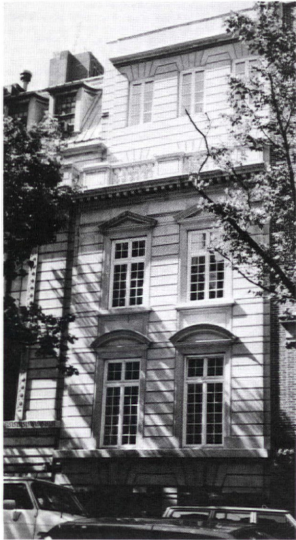
The new Indiana limestone facade as construction is being completed. Carved stone elements are set in a thin mortar bed — and held to the front wall with stainless steel anchors
