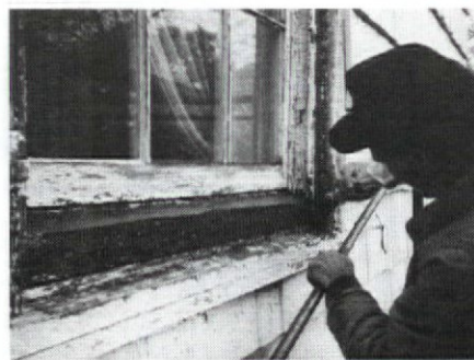
Craftsman from CONSERVATION SERVICES applies epoxy repairs to a badly deteriorated windowsill and frame. Write in No. 175
