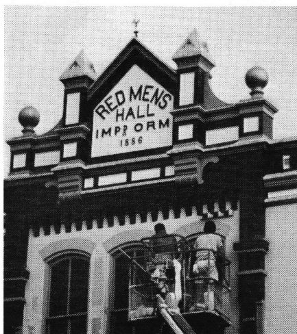
■ Restoration of facade, in Mount Holly, N.J., included pressure washing, painting (ten colors!), marblizing, and rebuilding wood lintels. Expertise includes custom signmaking of all kinds; scale drawings; historic jobs a specialty. Musgrove Graphic Design , 209 High St., Dept. TB, Mount Holly, NJ 08060 (609) 267-3393. Write in No. 765
