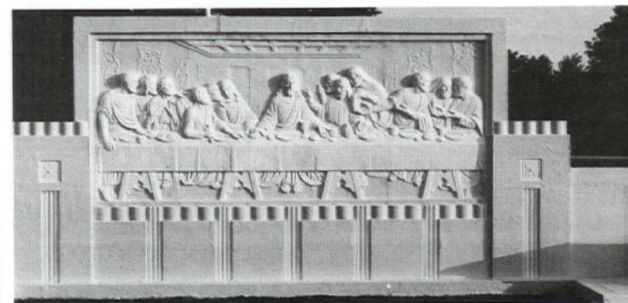
Deteriorated cast concrete bas-relief sculpture was restored with epoxies by Creative Sculpture Design & Restoration
