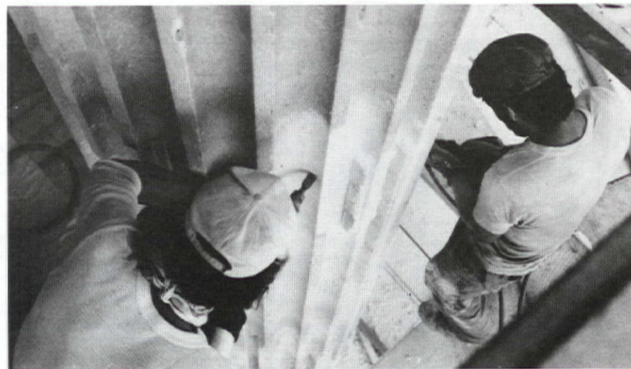
Carved marble "Dutchmen" inserted into damaged Georgia marble columns by craftsmen from Pietra Dura during restoration of Brooklyn Borough Hall
