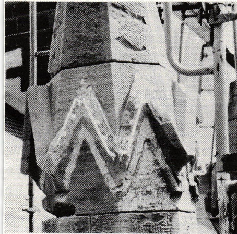
Workers remove deteriorated stone using hand-held hammers and chisels along with the same pneumatic carving heads they use to rake mortar joints for repointing. They then drill the stone wherever armatures will be required.
