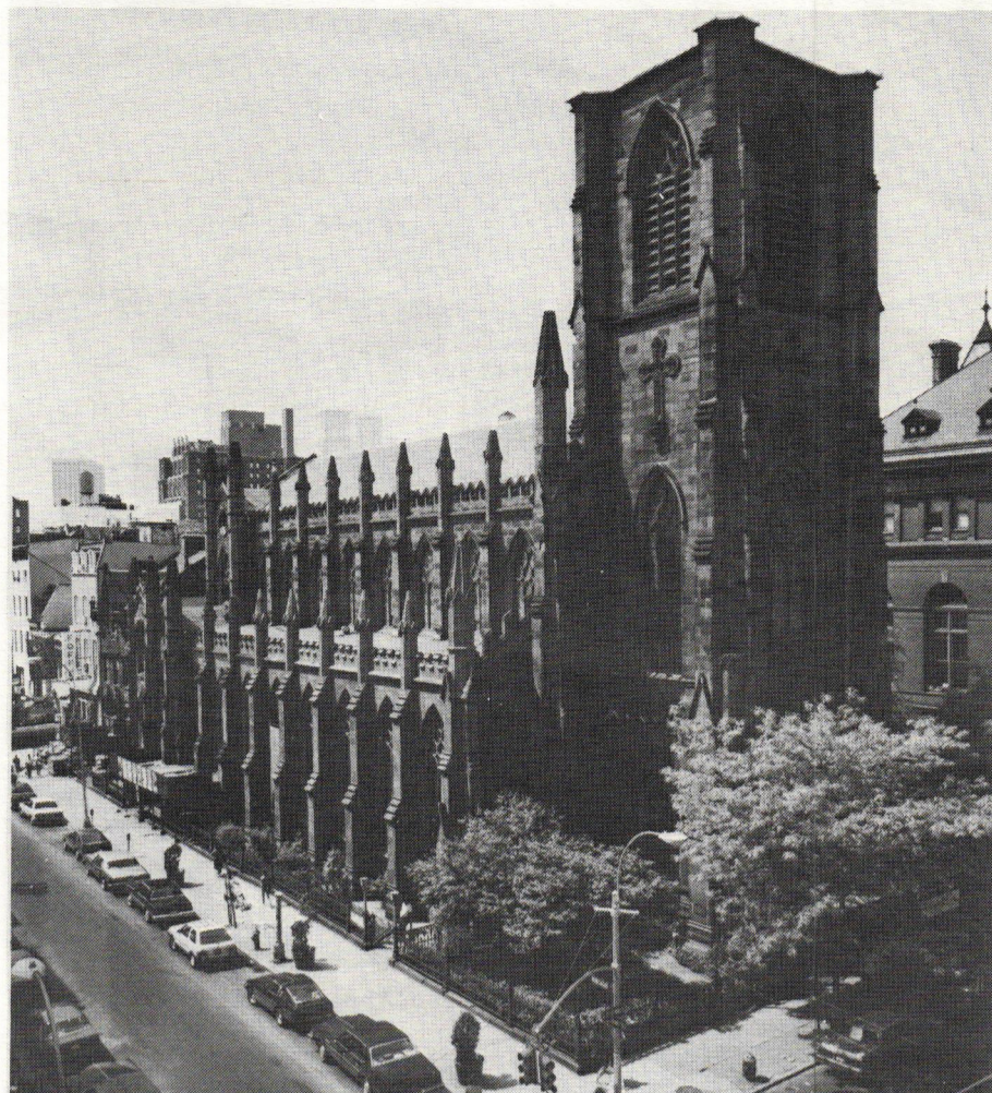
The Church of St. Ann and the Holy Trinity (1847) has lost, among other things, its original 100-ft. spire and numerous crockets and finials because of sandstone deterioration.
