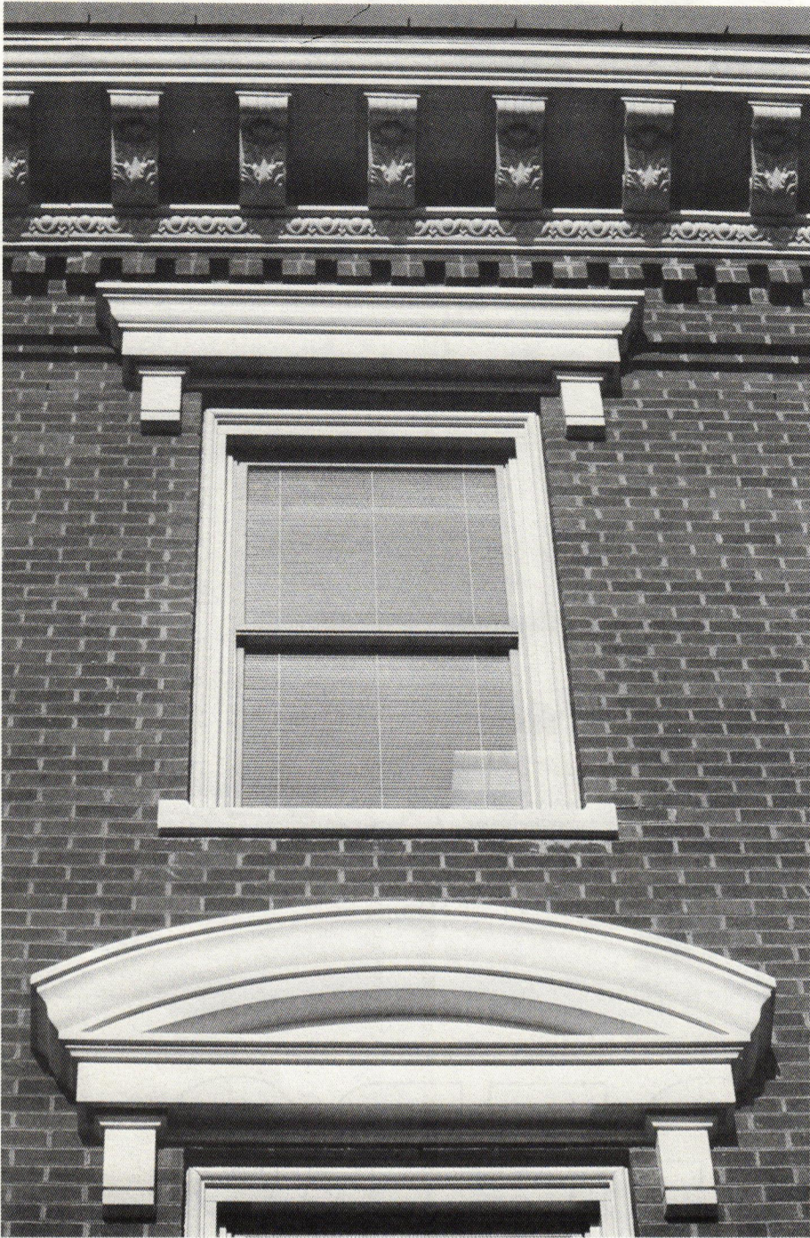
For this exterior restoration, window hoods and cornice were replicated in white FRP by FIBERTECH CORP.
