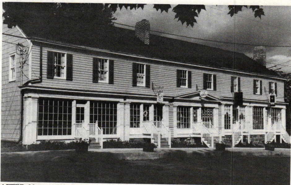
AFTER: New wood windows, storefronts, and millwork were custom-produced to Meadows' drawings by Millwork Specialties of Brooklyn, N.Y., preserving the traditional character of the building.
