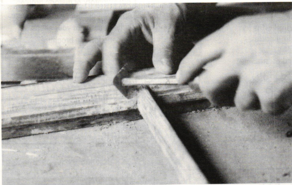
Sash was taken to the shop for quick repairs. Glass was removed, and all loose paint and putty carefully stripped with scrapers. After repairs, the sash was re-glazed with the original 1/4-in glass. Next day, when the sash was put back into the window frames, integral brass weatherstripping was also installed.
