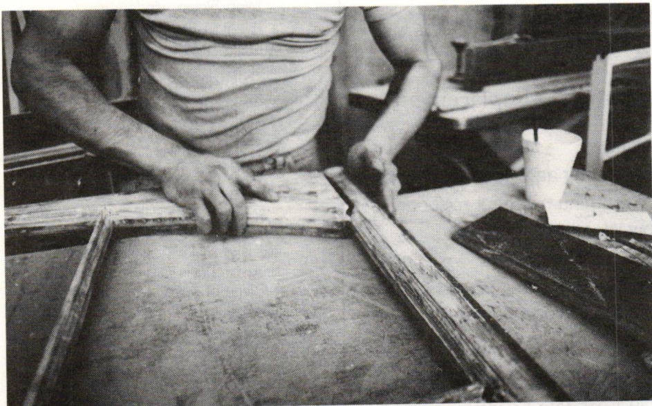
Loose joints were taken apart, glued with epoxy, and repinned. Rotted or damaged wood was restored with epoxy consolidant and filler. When an individual rail was beyond repair, a new "dutchman" was spliced in. If more than 35% of a sash was beyond repair, a whole new sash was manufactured.
