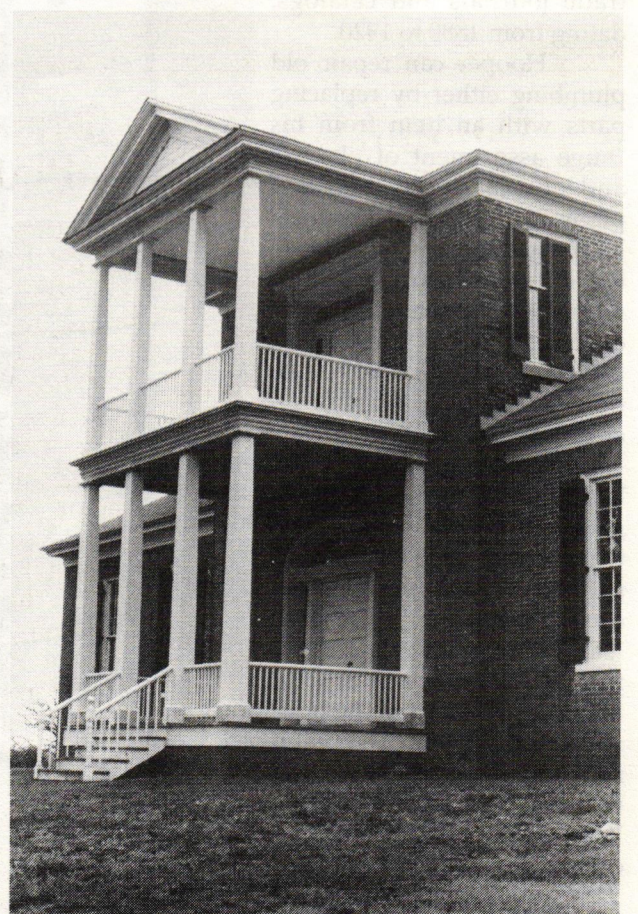
The Belle Mont portico was pulled back from the brink of collapse. Wherever possible, original material was kept — and repaired or patched as necessary.
