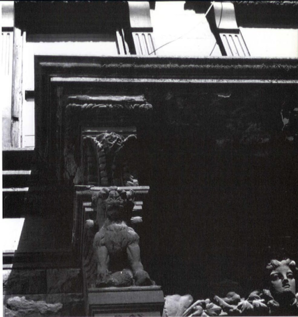
Punchlist teams document the condition of buildings that face — and have a visual impact on — public spaces.
