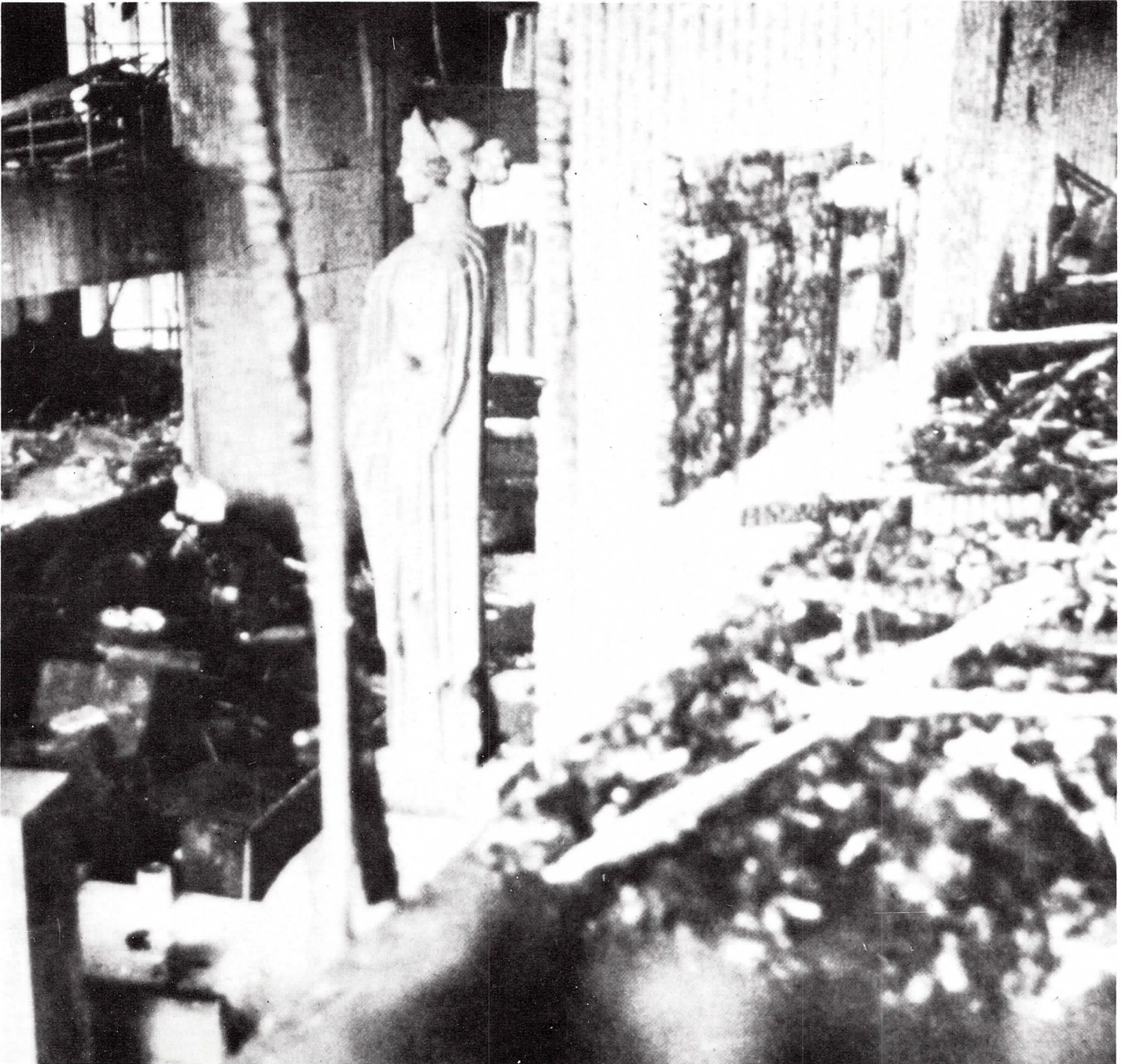
Figure 35. Art and Architecture Building, Yale University, New Haven, Connecticut. Paul Rudolph, architect, 1963. After the fire of June 1969.
