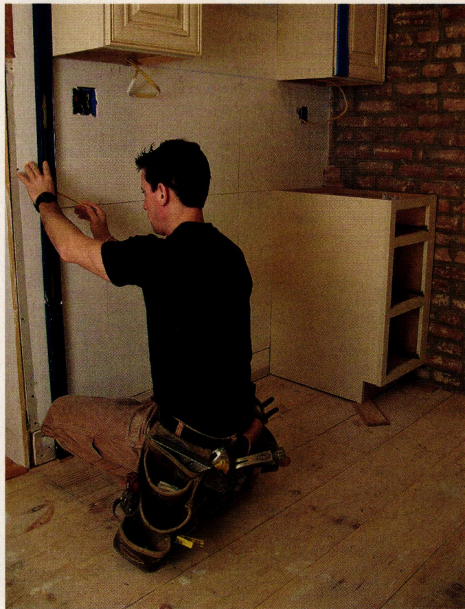
ABOVE: Base cabinets need to align with the uppers completely. Here, Mark plumbs down from the installed upper cabinet to line up the position of a stand-alone base. The stove will sit between this base and the corner unit, so he also measures the front opening to be certain it will fit.
