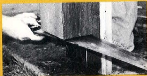
10" rotted bottoms of these load-bearing columns...
