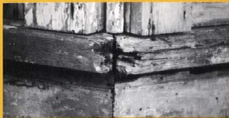
This rotted – and irreplaceable – woodwork...
