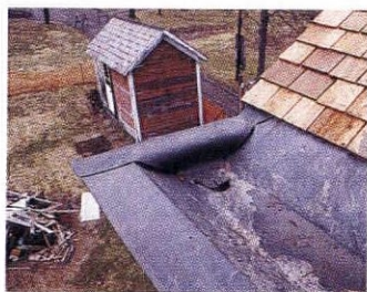
Rubber is not a historic material, but it's not visible from below, and it has a proven track record for box gutters.
