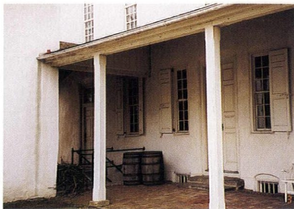
Stains on this stucco house are evidence that water is dripping down the wall, and very likely getting inside.
