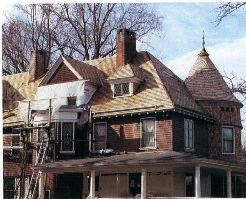
Incorporated into this hipped roof are a gable dormer and a hipped dormer, as well as a conical tower. Note, too, the eyebrow set in the hip.
