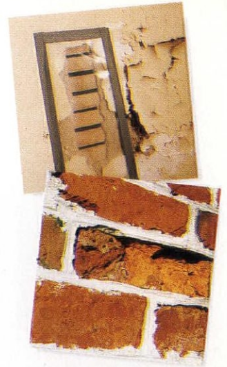
Sheet plastic (top) will detect general moisture presence and location when condensation appears on one side. Spalling brick (above) is a visual clue to high-moisture levels.
