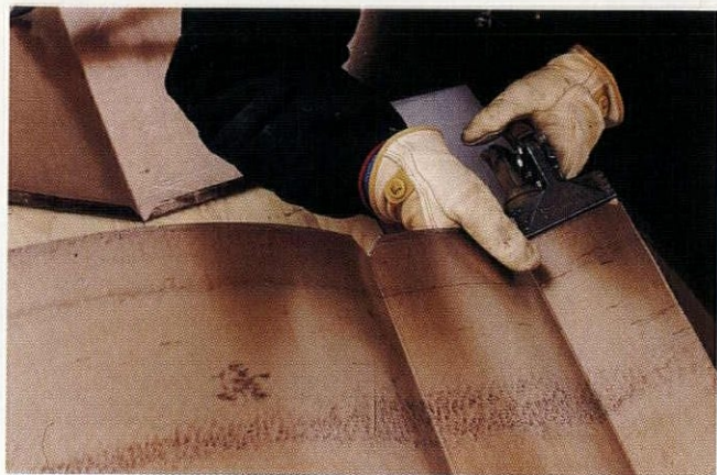
To form the lock seams, cut triangular notches at the folds and then bend the edges as needed with a hand seamer.
