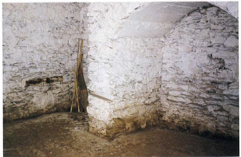
This 1743 basement is clay, packed almost as hard as rock, but extremely porous. Underground moisture that evaporates into the house is often the No. 1 source of humidity.
