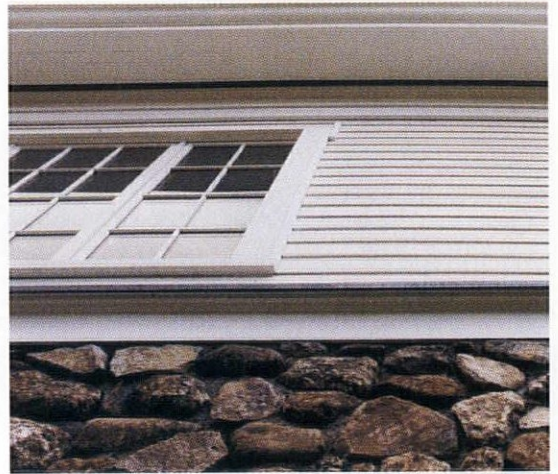
This house offers a good example of venting exterior walls. The dark lines where the wall meets the foundation and at the cornice are vents.
