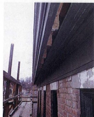
In addition to providing attic ventilation, soffit vents provide a quick exit from the cornice for moisture that leaks through the liner. This vent will receive insect screening to be lightly painted the cornice's green.
