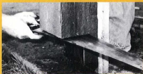
10" rotted bottoms of these load-bearing columns...
