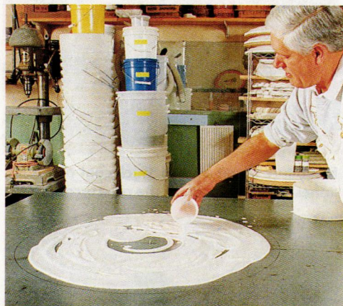
When ready, mix up plain gypsum plaster (plaster of paris) and apply it onto the board in a ring the size of the medallion.
