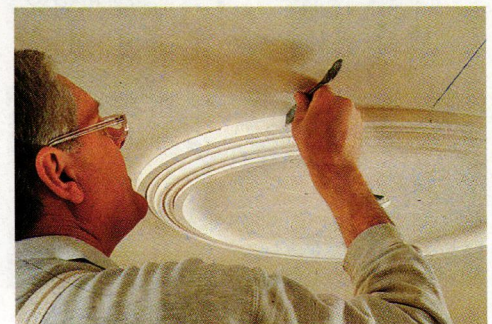
Apply plaster to seams with a paint brush as you might caulk around wood mouldings.
