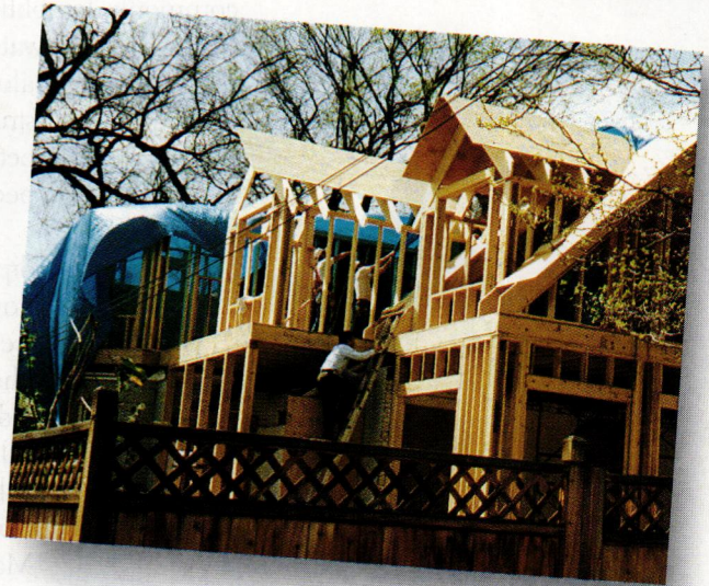
New construction on old houses requires many trades and someone to orchestrate the job.
