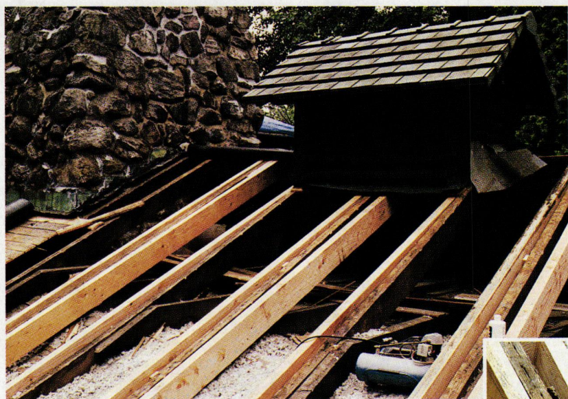
ABOVE: The kitchen rafters had spread worst at the middle of the roof — so much so that they affected how the roof tiles drained. Sistering with 3 x 8 lumber reinforced each rafter with identical material, but was not intended to correct the sag. INSET: The sisters stopped short of the original rafter tails, which were restored with epoxy fillers.
