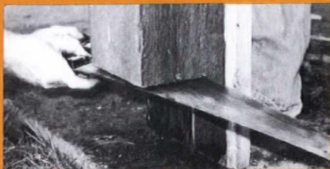
10" rotted bottoms of these load-bearing columns...
